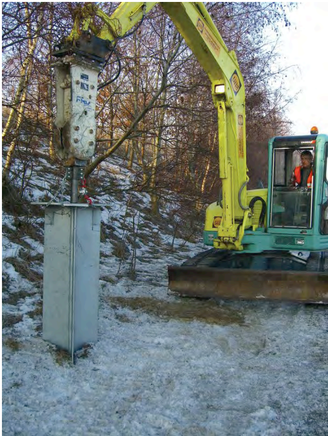
GroundPlug being driven into the ground prior to fixing of the sign assembly.
