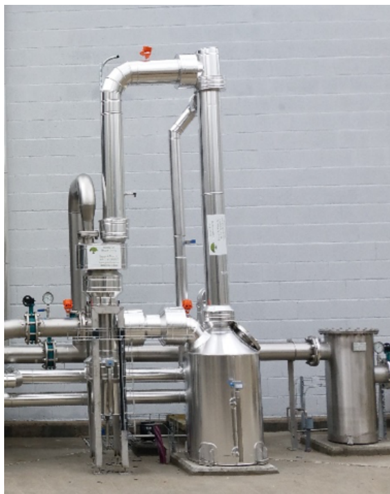
Figure 2. Biogas drying system/water vapor removal facility developed by Energy & Waste S.l group. Vertical position of the heat exchanger with heat recover system. Located in Alcala Oeste WWTP-Madrid Spain.
