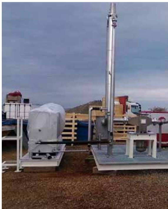
Figure 1. . Biogas drying system/water vapor removal facility developed by Energy & Waste S.l group. Vertical position of the heat exchanger. Located in Albufera WWTP-Valencia Spain.
