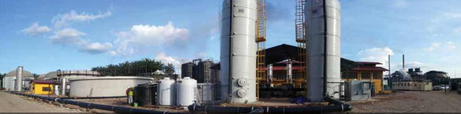
Piping and System Integration including Scrubber, Dryer and Booster to 4 units of 1MW Engine
