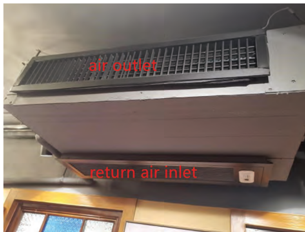
Figure 1. Inlet and outlet of air conditioner described in study of COVID-19 outbreak associated with air conditioning in restaurant, Guangzhou, China, 2020 (2).
