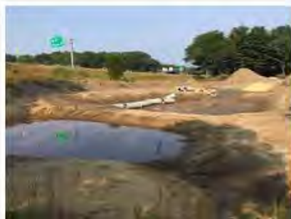
A roadside pond is being constructed next to Route 2 West by Exit 52A to collect and treat stormwater runoff.
