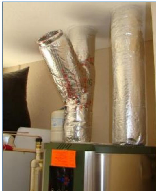
Figure 37. Y-type ducting arrangement at Site 5 allowing cold exhaust air to be diverted from the conditioned living environment
