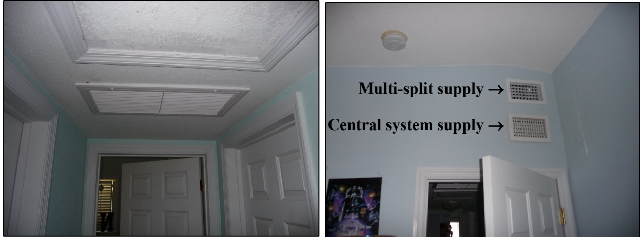
Figure 14. Ceiling-mounted fan coil return grille (left); existing and new supply registers (right)
