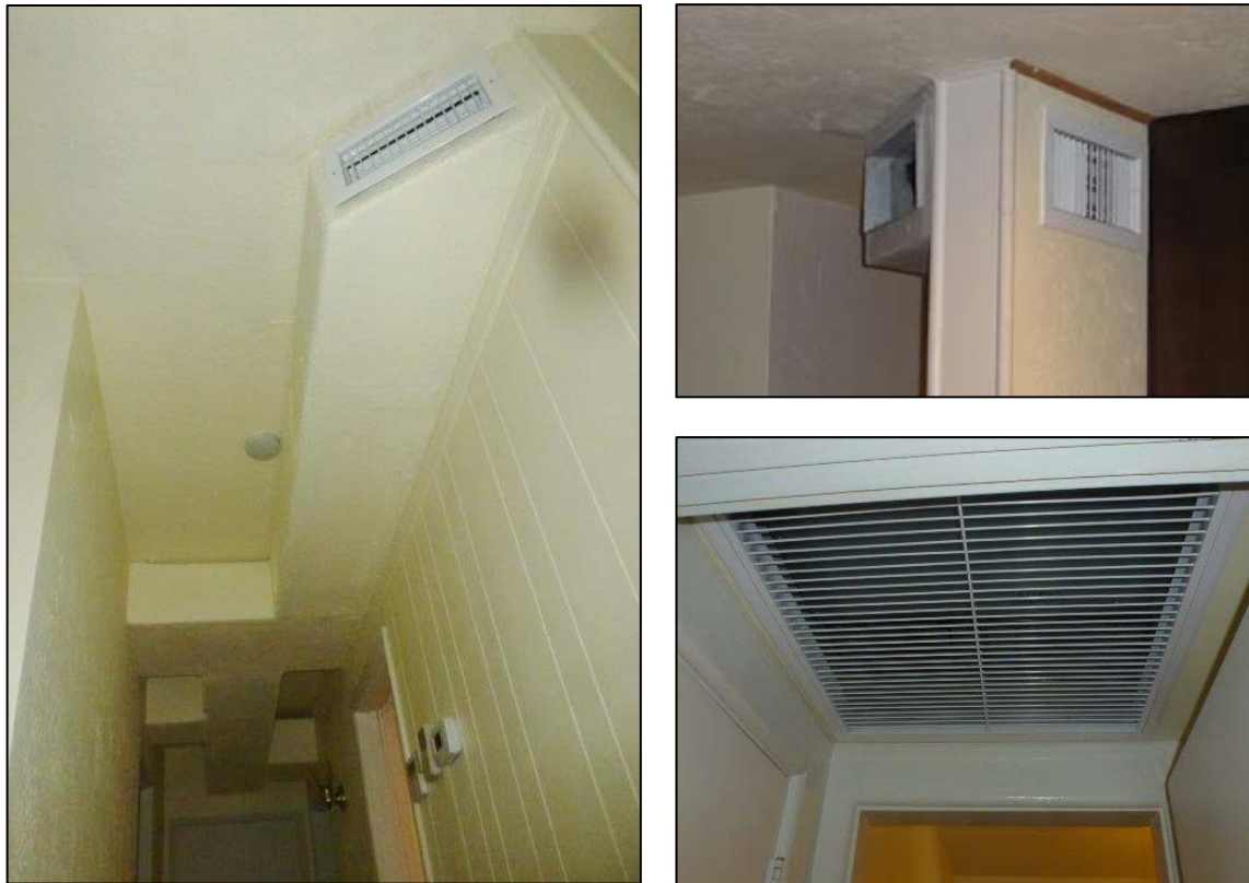
Figure 26. Finished ducted MSHP installation: ductwork (left and upper right) and fan coil (lower right)
