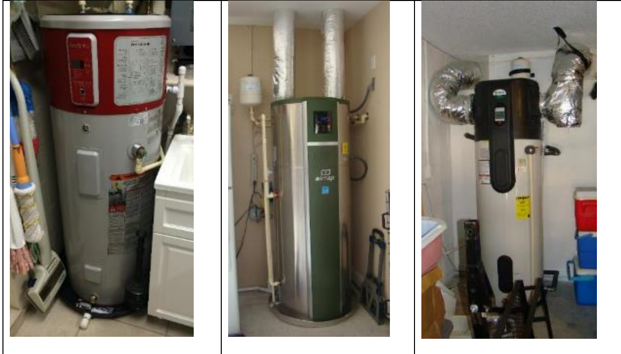
Figure 30. HPWH configurations: interior GE unit in utility room at Site 13 (left); ducted Air Generate unit at Site 5 (center); ducted A.O. Smith unit at Site 26 (right)
