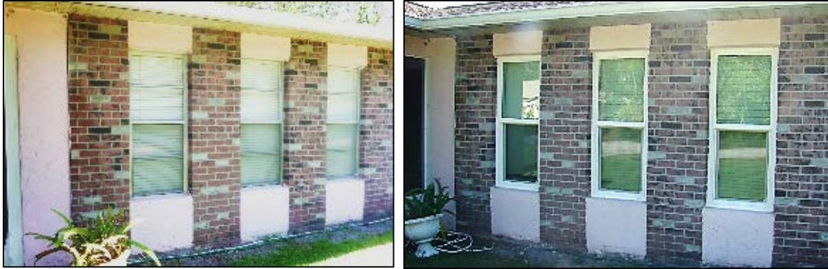
Figure 48. Window retrofit for Site 23: pre-retrofit with existing single-pane, metal-framed windows (left); post-retrofit with double-pane, vinyl-frame windows (right)
