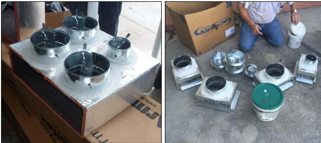
Figure 11. Dampered collars for four supply ducts attached and sealed to fabricated junction box (left); supply register boots sealed with mastic (right)
