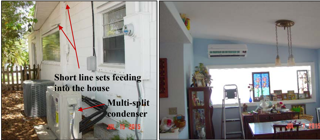
Figure 9. Condenser location, nearby electrical panel, and short exterior line set runs (left); centrally-located, wall-mounted fan coil (right)
