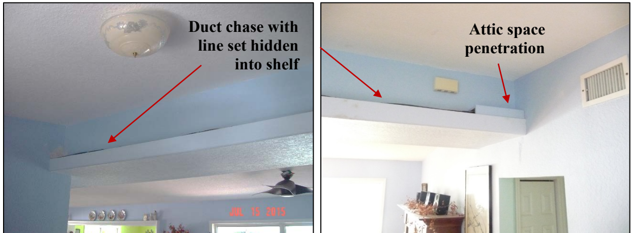
Figure 15. Line set tucked into the existing central system duct chase shelf
