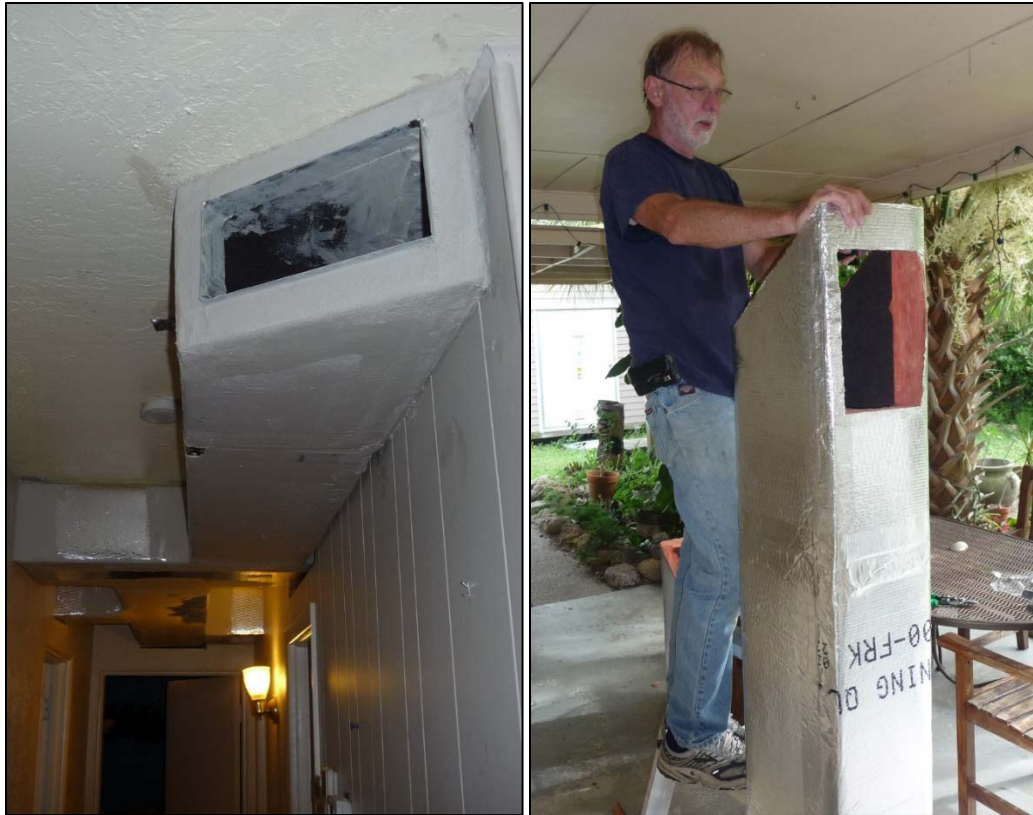
Figure 24. Construction of living room and kitchen supply air duct (left); fabricated ducts installed and sealed with mastic (right)
