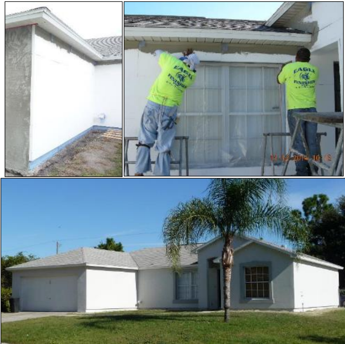
Figure 41. Attachment of 2-in. polystyrene insulation (top left), final textured coat application (top right), and completed EIFS retrofit (bottom) for Site 54
