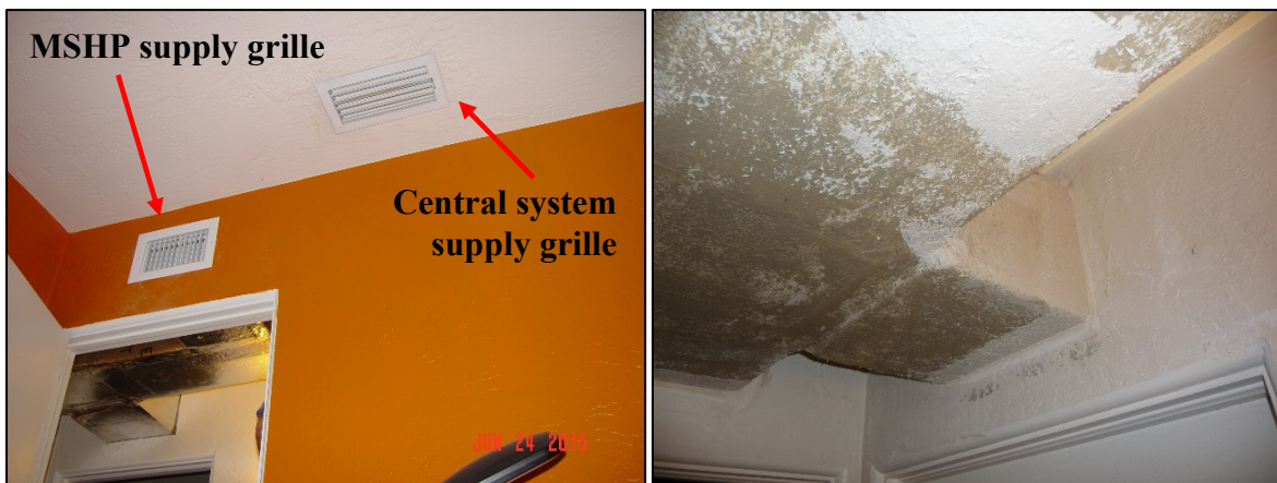
Figure 25. Bedroom view showing both the MSHP and the original central system supply grilles (left); sealed wall penetrations (right)
