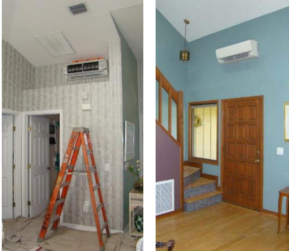
Figure 2. Wall-mounted MSHP fan coil at Site 3 and Site 24
