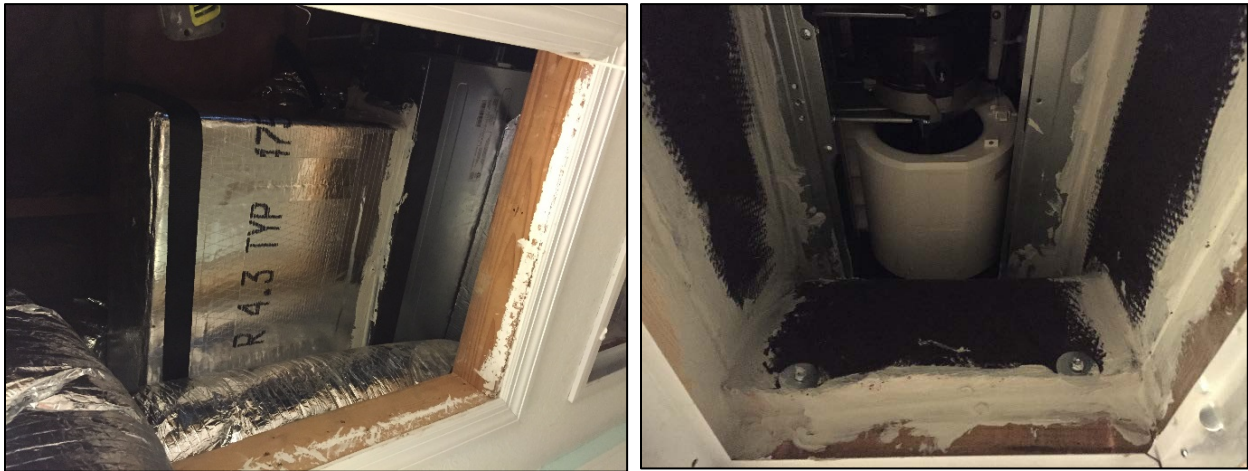
Figure 13. Fabricated junction box installed above attic hatch (left); return plenum and mini-split fan coil installed above ceiling penetration with seams sealed (right)
