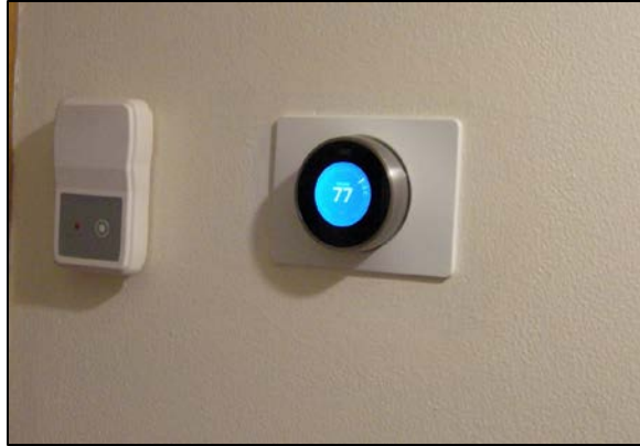
Figure 74. Installed Nest and broadband temperature and RH measurement by thermostat at Site 16
