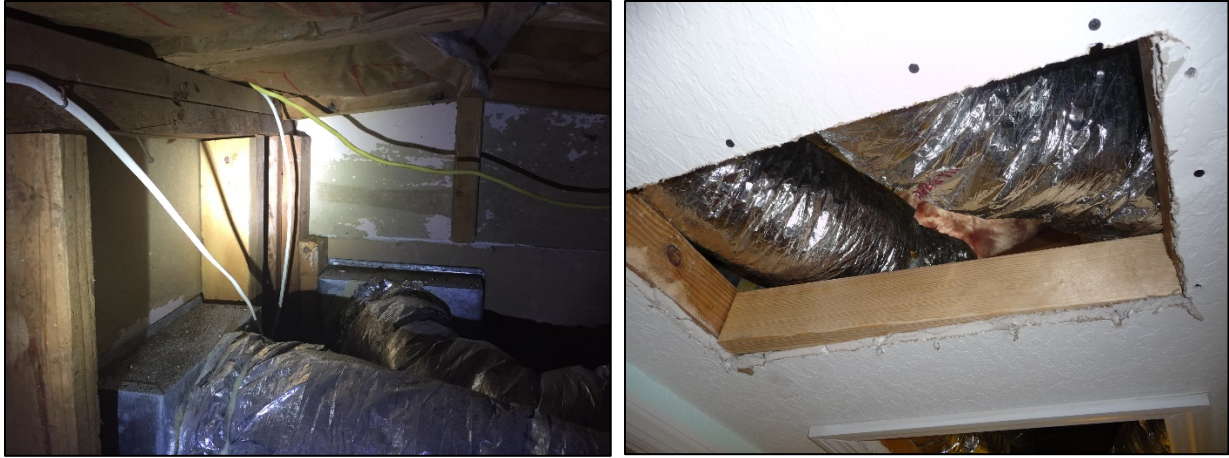
Figure 12. Pre-retrofit attic space used for the ceiling-mounted fan coil and supply air ducting (left); penetration into attic to mount the air handling unit (right)
