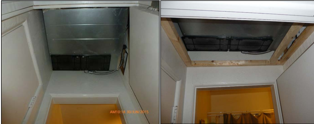
Figure 22. Looking up at installed fan coil unit unframed (left) and framed (right)
