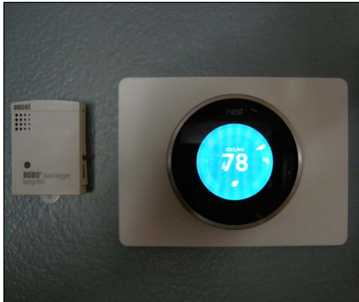
Figure 63. The Nest learning thermostat installed at one of the PDR sites showing the redundant temperature and humidity measurement
