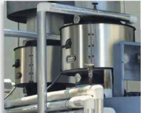
Industrial Laundry, Fresno, California (2) EM Series, boiler economizers, preheating boiler feedwater for (2) 115 BHP Parker steam boilers.
