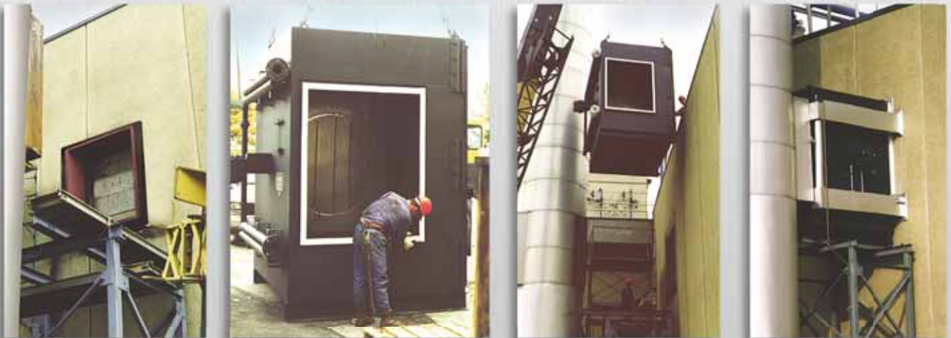
Brewery, Ontario, Canada (1) RTR-1V2Q28CSS recovering Btu from (1) 95,000 pph steam boiler; Reducing 505°F @ 24278 SCFM to 333°F; Raising 196 gpm boiler feedwater entering at 225°F to 278°F.
