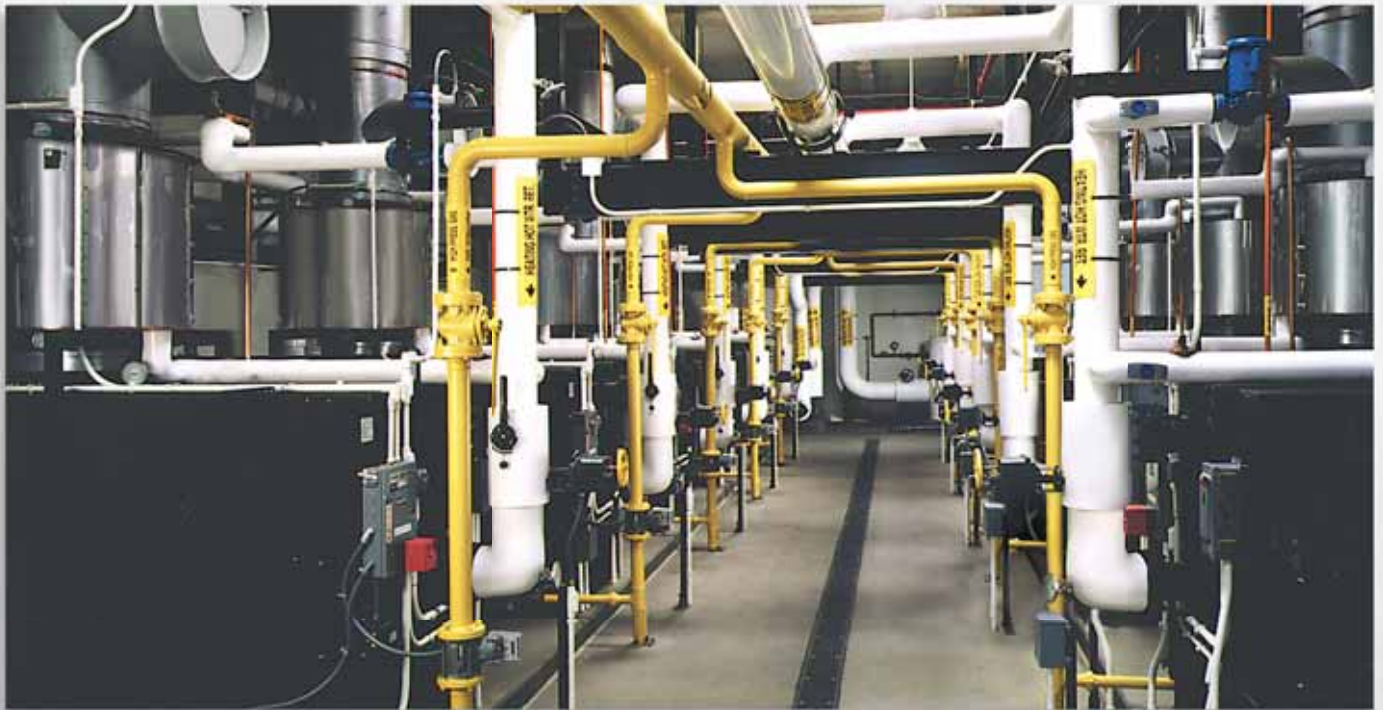
College Campus , Long Beach, California (10) EM Series boiler economizers preheating hot water return loops.
