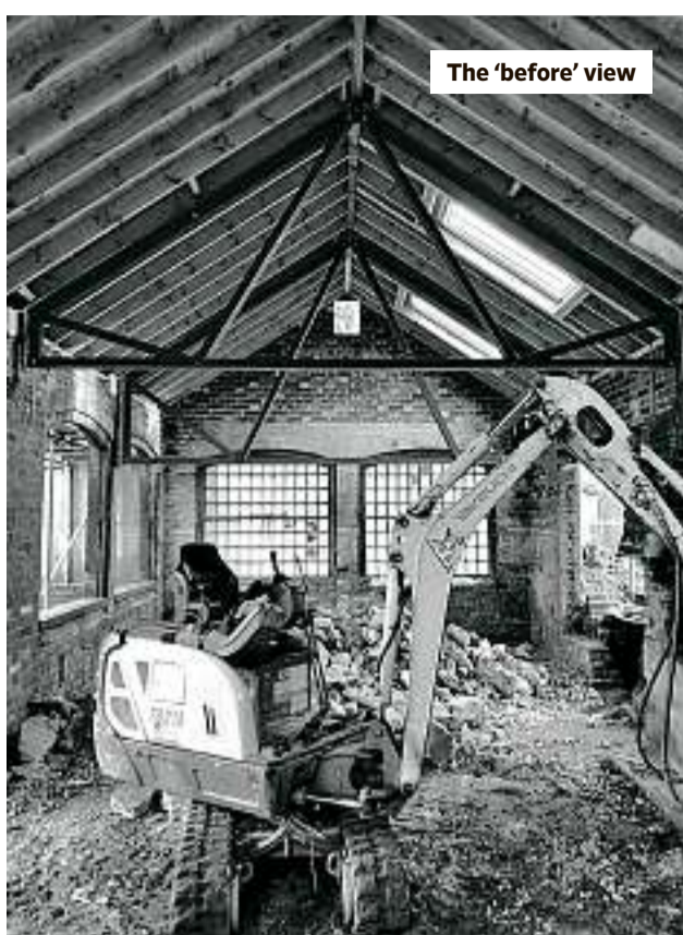
The forge was being used as a substation when the Grundys bought it. It required extensive work.
