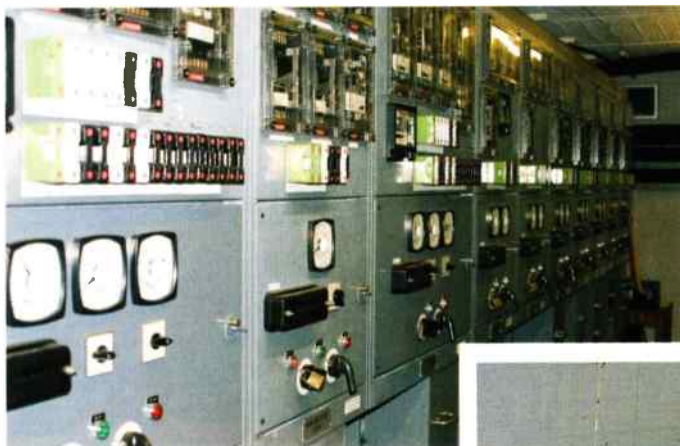
● This is definitely not a room for the faint hearted. The 11kV switching room. The contactors which are used to power the selected senders are very loud when operating. Similar in level to a large calibre gun shot.
