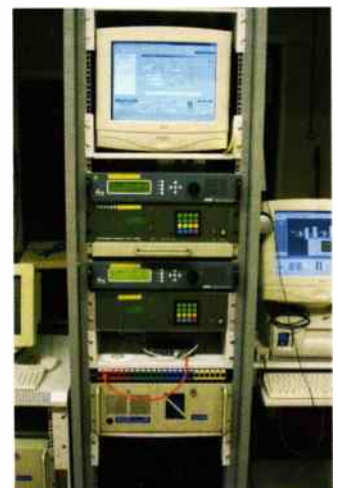
● DRM Control, modulation and monitoring rack.
