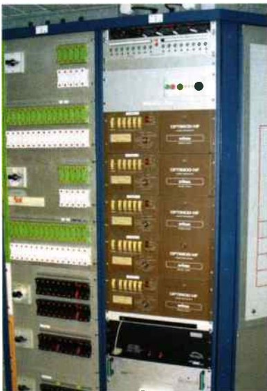
● The rack of Optimod 9105A audio processors used for programme feed enhancement prior to feeding the modulators.
