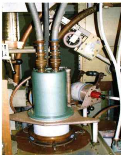
● A Thomson TH558 tetrode p.a. valve in-situ inside Sender 45.
