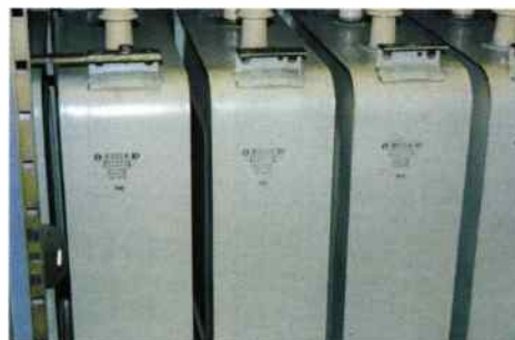
● A bank of 2 \mu F 31kV capacitors located in the modulator section of Sender 45.
