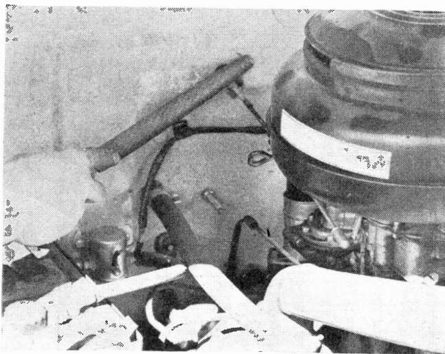
Poor ground connections on cables and rods which pass through the firewall may be quickly located by shorting them to the wall.
