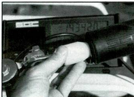
The large white insulator is necessary to prevent an arc-over at 2 MHz-6 MHz frequencies.
