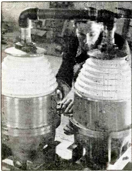
The WHAS transmission line end seal during the 1940's.
