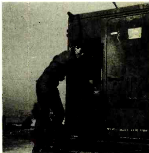
A shot of me in the "good old days"(?! ) connecting a power cable to a comm shelter in Korea.
