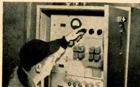
General Electric engineers, working closely with AL personnel, developed and installed the control systems which regulate the mill.
