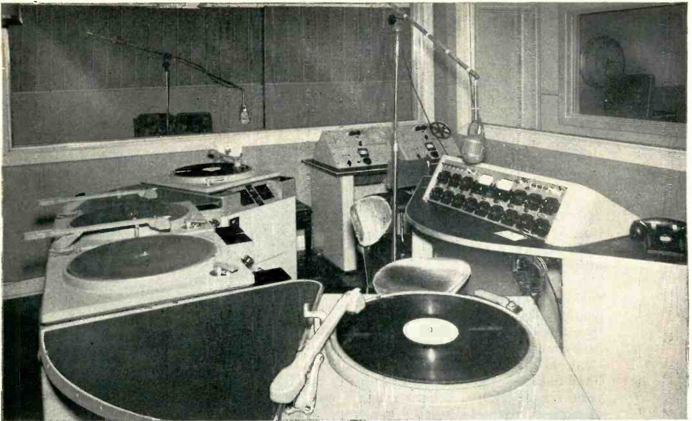
Control Room WGEM, Quincy, Illinois Affiliated with GATES
