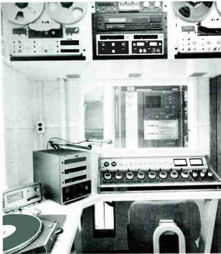
Internal view of mobile studio with FM-3.5A transmitter visible in background.
