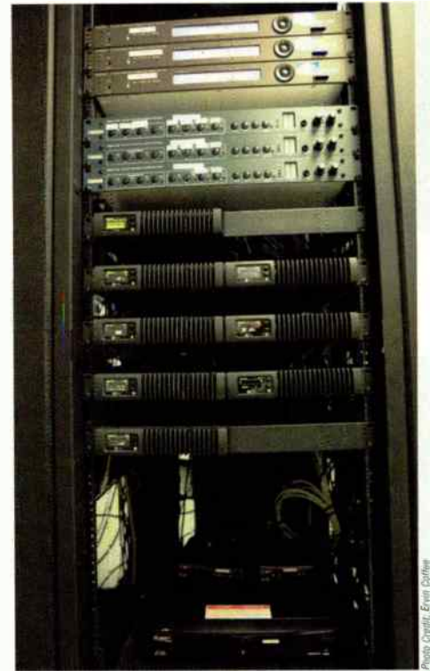
One of many racks in the CPR facility holds DEVA 8008 silence sensor/backup audio players, Broadcast Tools ADMS 44.22 analog/digital matrix switchers and Axia xNodes.
