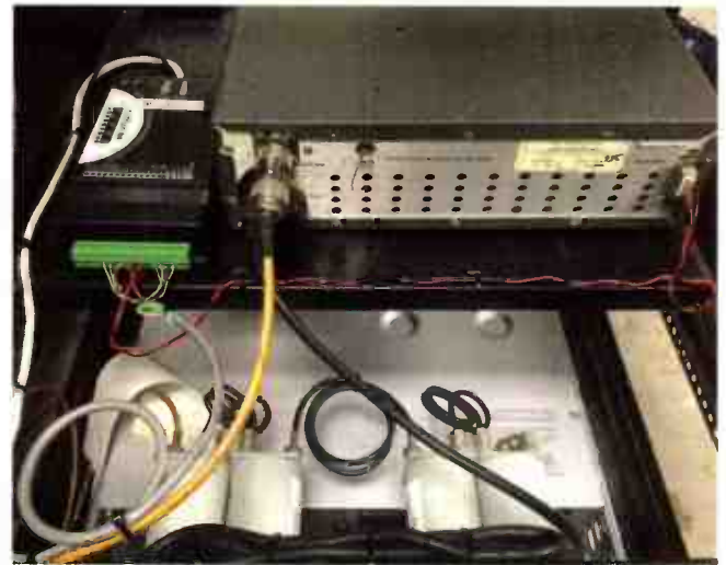
The Broadcast Tools I/O Sentinel, seen at left, allows the remote keying of the Marti TX by way of a GUI on the rack room remote control.
