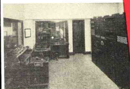
Principal units of the central speech-input control room. Brand new RCA high-fidelity equipment throughout.
