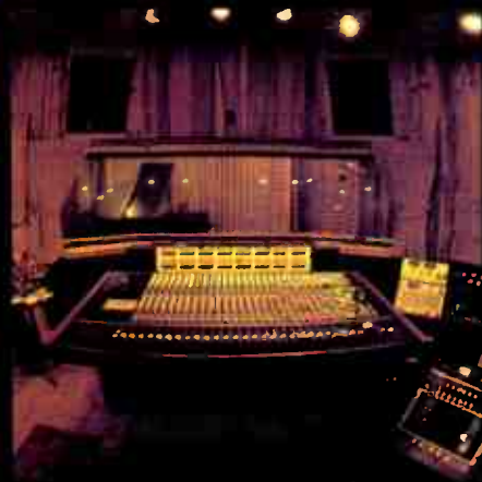
CONTROL ROOM B
