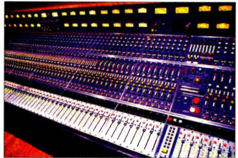
Coast Recorders' custom Neve 5305 console was created from two identical (and consecutively numbered) 5305 consoles originally built for Yorkshire Television. The 72-input all-discrete console features GML automation. Modifications by Dan Alexander Audio.
