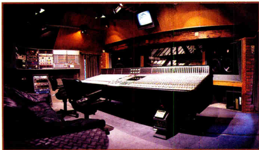
The control room at Ridge Farm Studios has a new SSL 9000J console, installed this summer.
