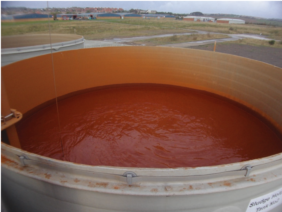
Fig. 3.10 Sludge collection tank of the former active Horden mine water treatment plant (County Durham, England, United Kingdom)
