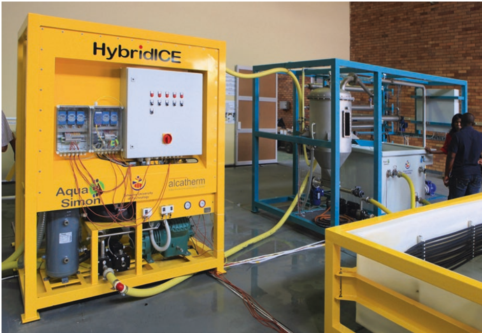
Fig. 3.32 Former water treatment plant for eutectic freeze crystallisation at the Soshanguve campus of the Tshwane University of Technology, Pretoria, South Africa. (HybridICE® process)
