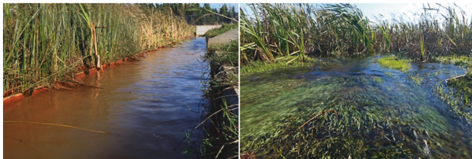
Fig. 4.9 Inlet (left) and outlet (right) of the aerobic constructed wetland Neville Street (Cape Breton Island, Nova Scotia, Canada). Water flows into the constructed wetland in an ochre and metal-rich state (left) and exits in a crystal-clear state with a substantially reduced metal load (right)
