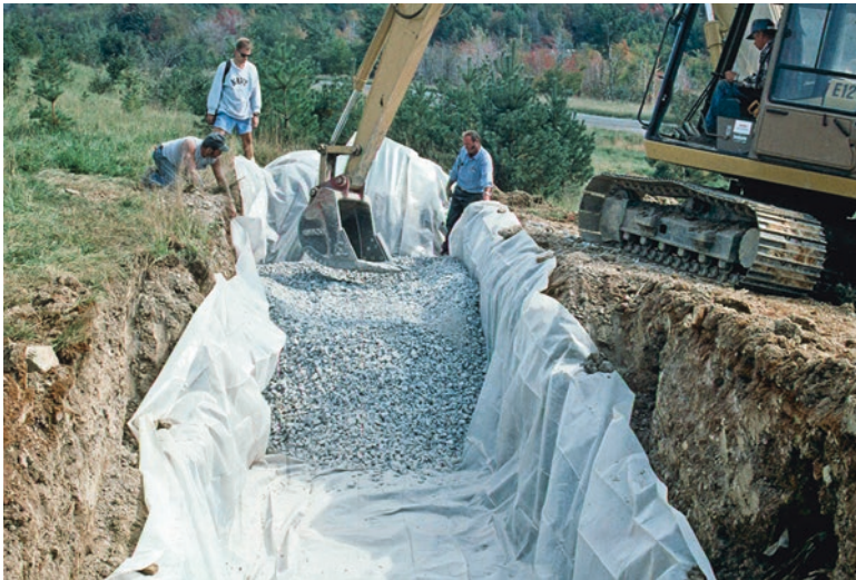
Fig. 4.5 Anoxic limestone drain during the construction phase. The liner sits in the open drain which is already filled with limestone at the rear end. (Photo: Jeff Skouson)
