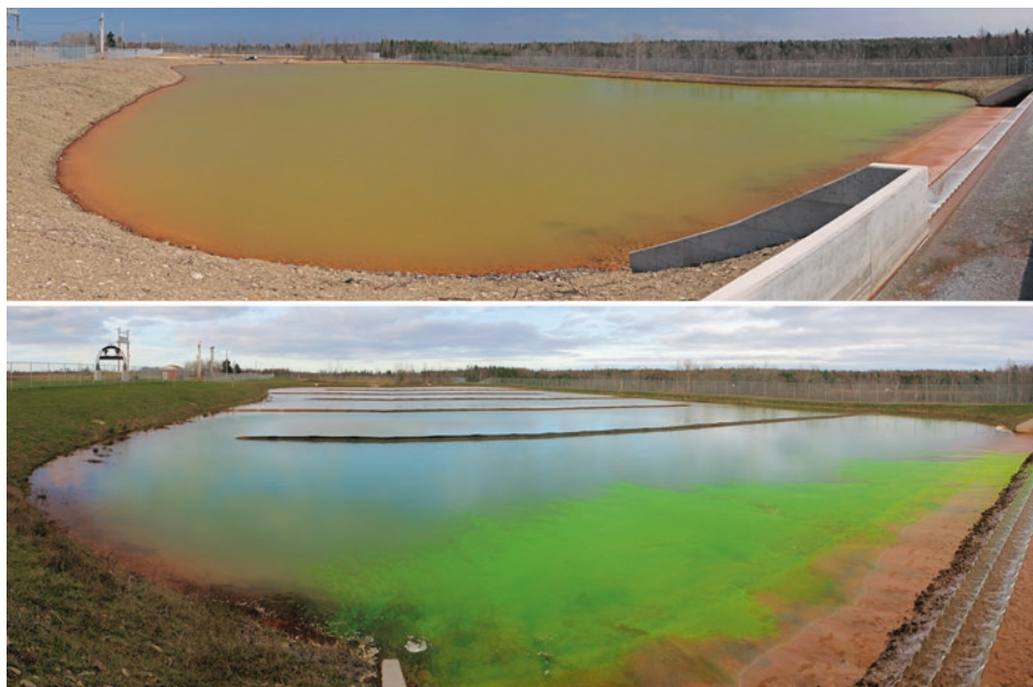
Fig. 4.16 Settling pond at the Neville Street passive mine water treatment system, Nova Scotia, Canada, before and after installation of baffle sheets. (Details in Wolkersdorfer 2011)
