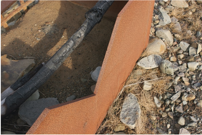
Fig. 2.11 Incorrectly constructed triangular weir for a mine water outlet of the 1 B Mine Pool on Cape Breton Island, Nova Scotia, Canada. The weir plate is too thick (2 cm), is made of non-stainless material, and lacks the sharp edge on the water side. The weir was in use for a period of about 1 year to measure flows with “high accuracy”
