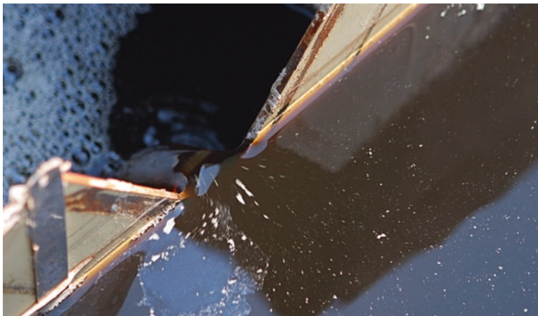
Fig. 2.10 Incorrectly installed measuring weir at the former IMPI pilot plant in Middleburg, Gauteng Province, South Africa. The sharp edge on the water side of the weir plate is missing
