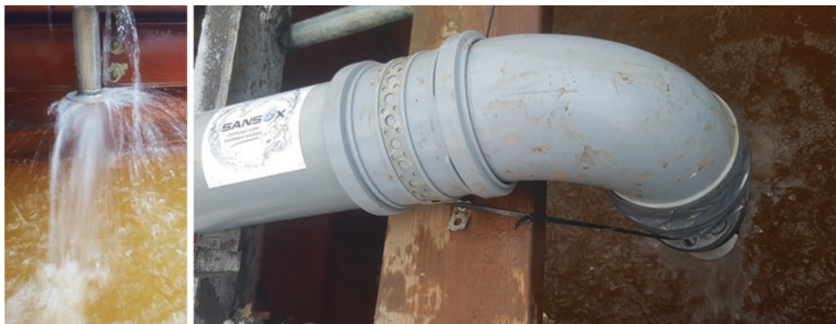
Fig. 4.25 OxTube in 90° angle installation on the Metsämonttu vertical flow reactor. The oxygen saturation in the mine water could thus be raised from about 40 to 60%
