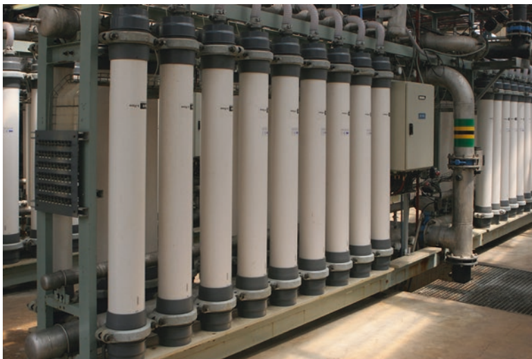
Fig. 3.18 Ultrafiltration unit of the eMalahleni mine water treatment plant in Gauteng Province, South Africa
