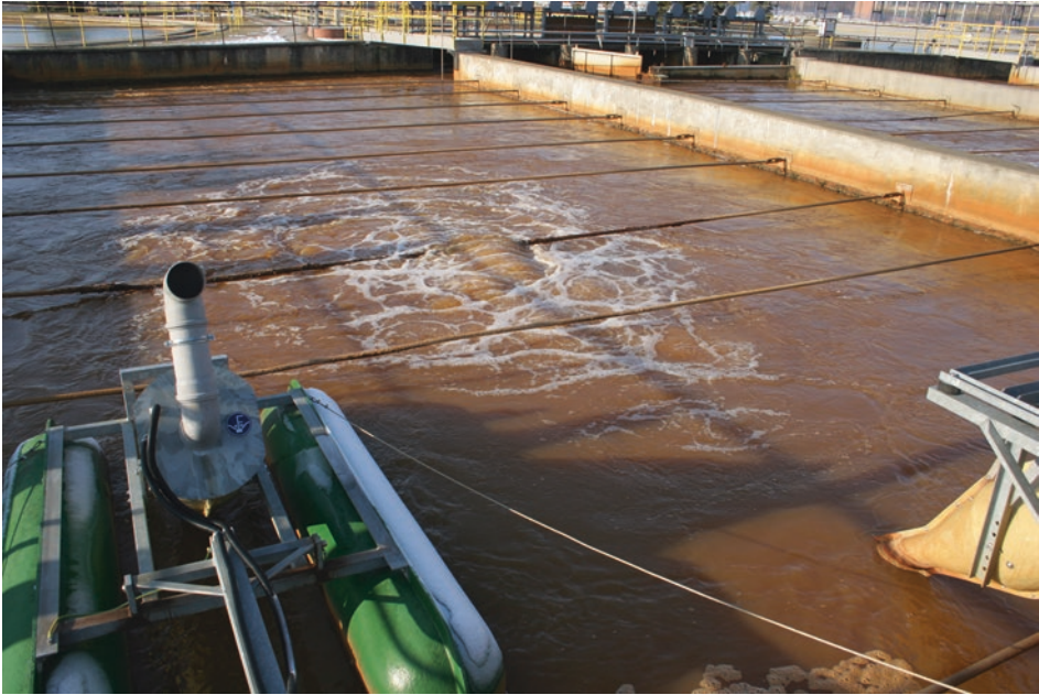
Fig. 3.7 Aeration of mine water in a low density sludge plant (mine water treatment plant Schwarze Pumpe, Lusatia, Germany)
