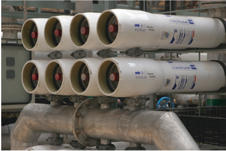
Fig. 3.20 Reverse osmosis unit of the eMalahleni mine water treatment plant in Gauteng Province, South Africa. (See also Fig. 7.7)
