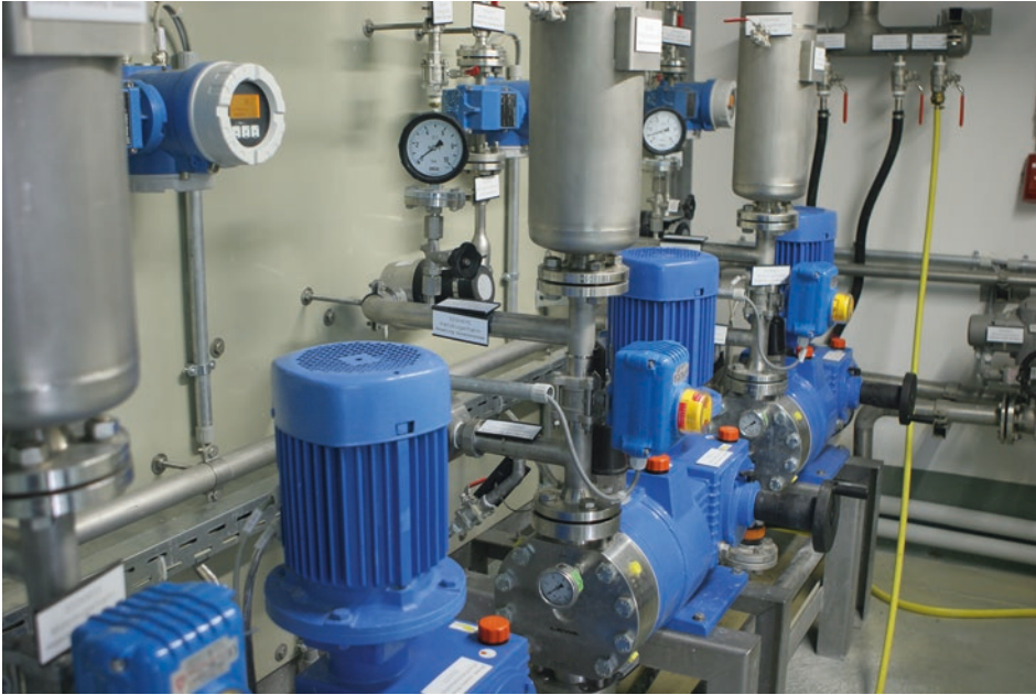
Fig. 3.2 Pumps for chemical feed in an active mine water treatment plant (Straßberg/Harz, Germany)
