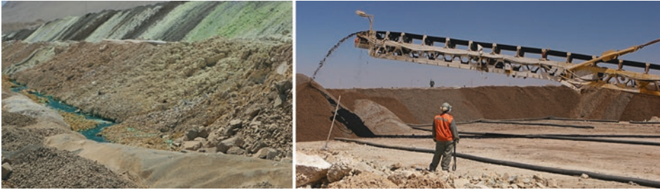
Fig. 5.4 Left: Collection trench of copper-containing solution from heap leaching; right: Preparation of a heap for microbologically assisted acid leaching of copper-rich ores (Chilean El Salvador copper mine of the Corporación Nacional del Cobre de Chile – Codelco)
