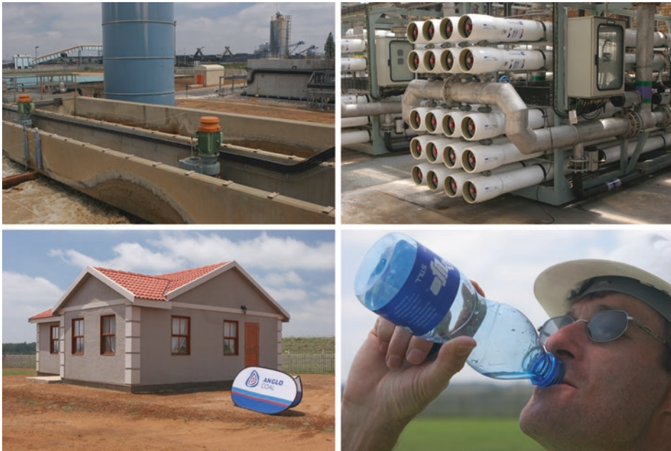
Fig. 7.7 Mine water treatment plant eMalahleni. From top left to bottom right: Pre-treatment (leaching basin in the background on the left and coal mine on the right); reverse osmosis; building made of gypsum; mineral water produced in the plant. (Gauteng Province, South Africa)
