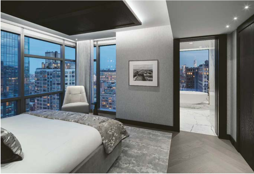
The tall needle skyscraper sways, so Rusk had to curtail its use of spinning lasers to level ceilings and millwork on windy days when the lines would move up and down the walls.
