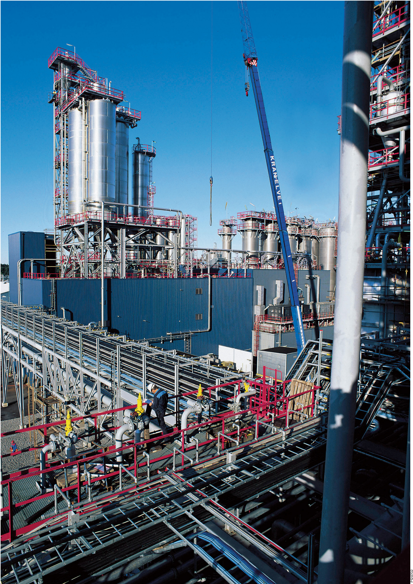
Wibe Cable Ladders KHZ and KHZP installed at Borealis Stenungsund. Borealis in Sweden supports customers with speciality plastics for some of the largest energy supply, oil and water pipeline projects in the world.
