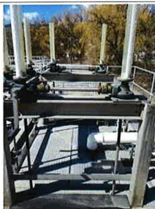
Primary Influent Splitter Gate
