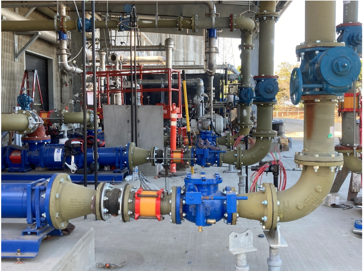
New Control Pumps and Piping for Digester 7
