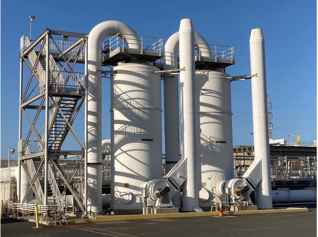
Aeriation Basin Order Scrubbers
