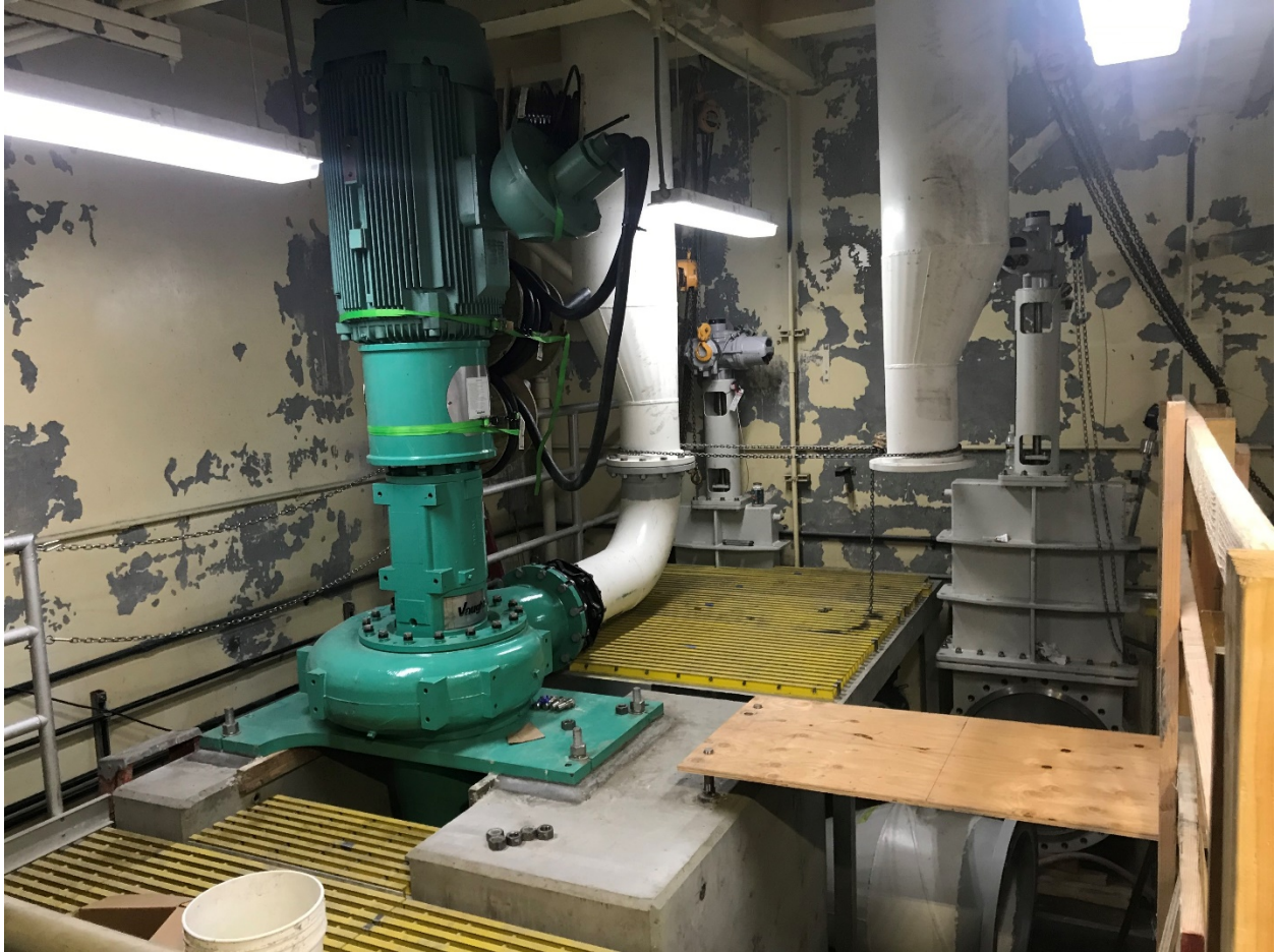
New Wastewater Pump, Piping and Gate Valve at the Alvarado Pump Station
