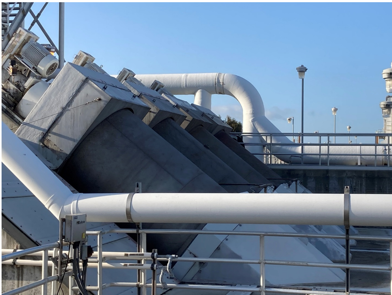
Primary Effluent Pumps for the Aeration Basin
