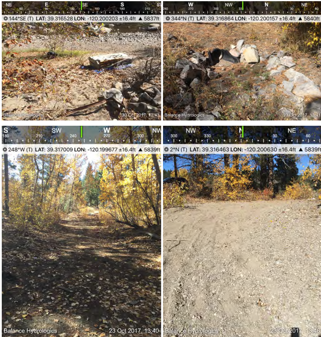
Figure 5-2 Donner Creek Confluence Site Existing Conditions. Top-left: Trash on river bank. Top-right: sediment build up at culvert. Bottom-left. vehicular path generates secondary flow path. Bottom-right: compacted vehicular access road.
