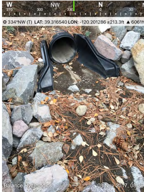
Figure 3-3. Sub-Watershed 1: Sediment Accumulation in Stormwater Culvert.
