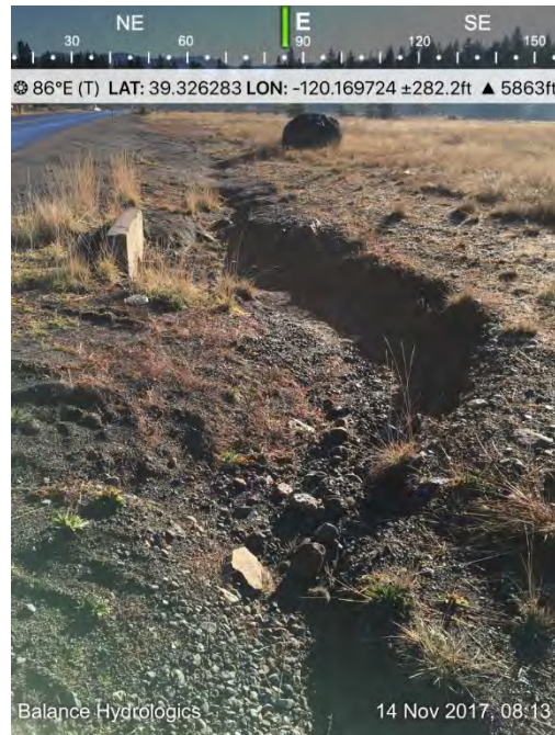
Figure 3-5. Sub-Watershed 17: Erosion at Estates Drive Culvert with Limited Downstream Treatment.
