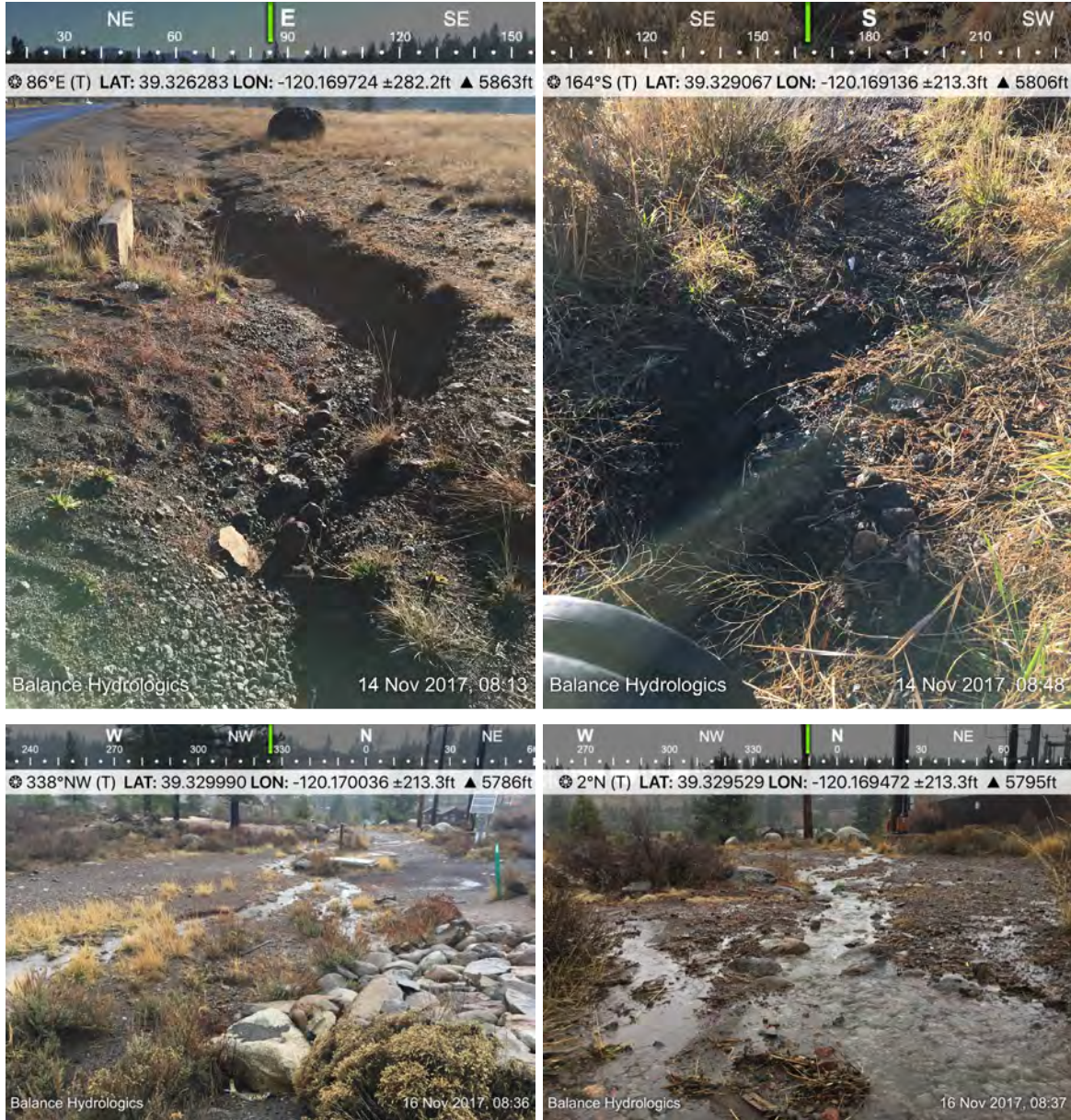
Figure 5-7 Estates and River View Drive Existing Stormwater Drainage Conditions. Top-left: Erosion along Estates Drive into culvert. Top-right: Erosion and path channelization at drain pipe inlet. Bottom-left: Stormwater draining and channelizing at the lower portion of Truckee River Regional Park, by the disk golf course. Bottom-right: Erosion and sediment from stormwater flows heading towards Truckee River.
