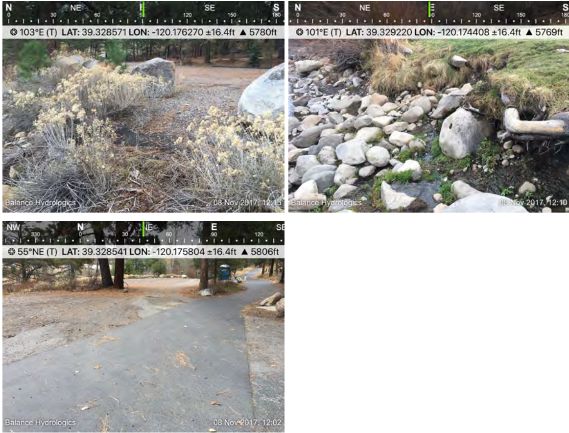
Figure 5-5 Truckee River Regional Park Riverside Parking Area Existing Conditions. Top-left: road material leaving parking area and towards slope above Truckee River. Top-right: Bank erosion along river access points. Bottom: Entrance to parking area along legacy trail.
