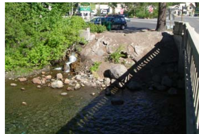
32. Existing culvert at Fanny Bridge could be improved with best management practices
