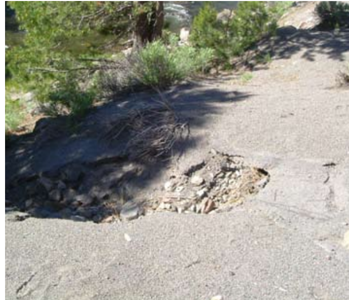
12. Poorly designed culvert draining highway is eroding bank into Truckee River
