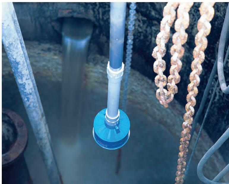
An ultrasonic level transducer measures the water level in a wet well.
