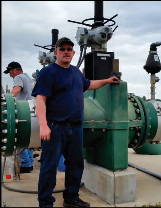
20" Onyx pinch valve handling raw waste water, Punta Gorda FL
