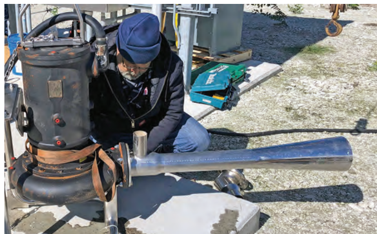
A Landia AeriGator chopper pump has helped resolve a lift station pump clogging problem in Madisonville, Texas.
