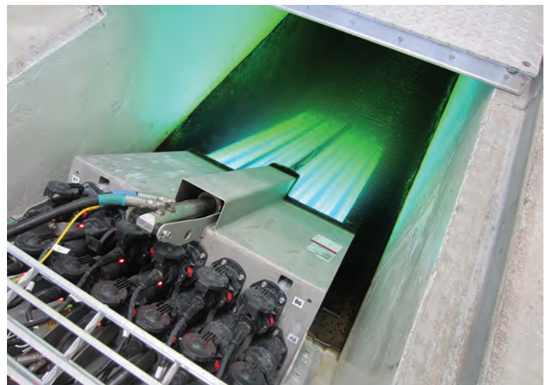
A TrojanUVSigna system disinfected the flow of wastewater.
