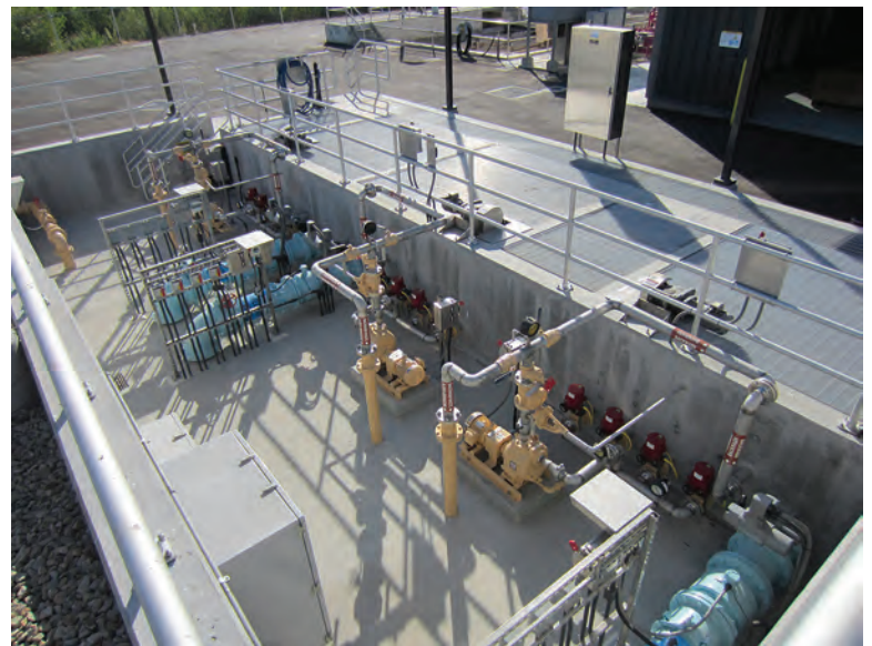
Paso Robles installed a cloth media filtration system (Aqua-Aerobic Systems) as part of an upgrade to tertiary treatment for water recycling.
