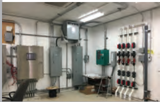
Control panels and alarms from Delta Treatment Systems'
