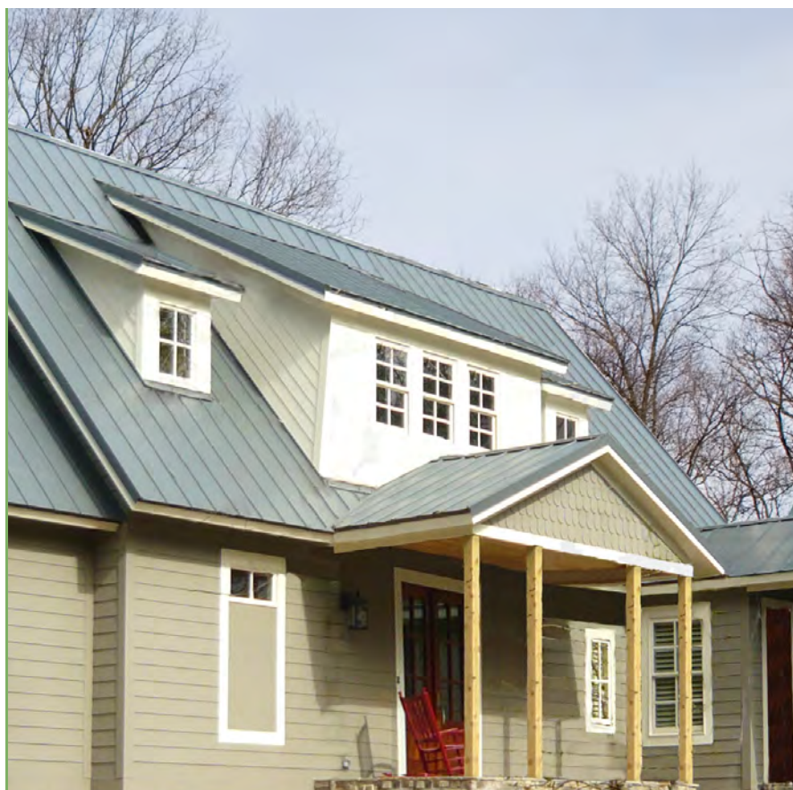
Horizon S in Charcoal Gray covers the roof of this home.
