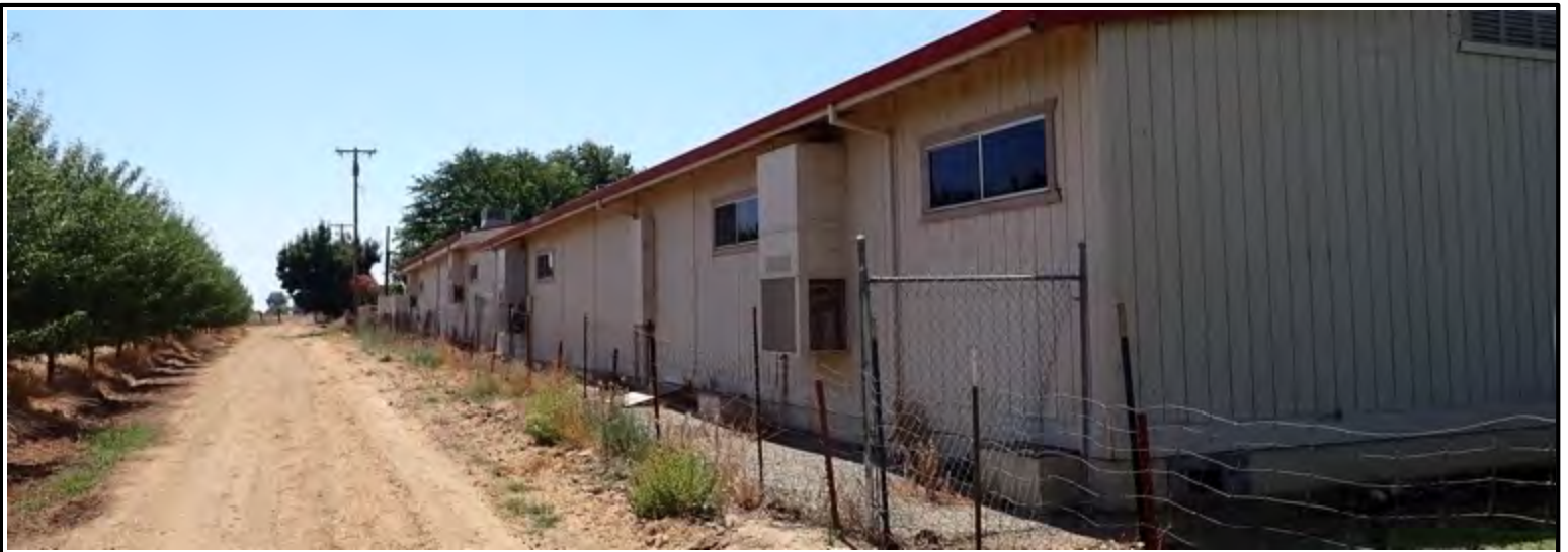
Image 4. Looking SW, four portable classrooms on the western side of subject property.
