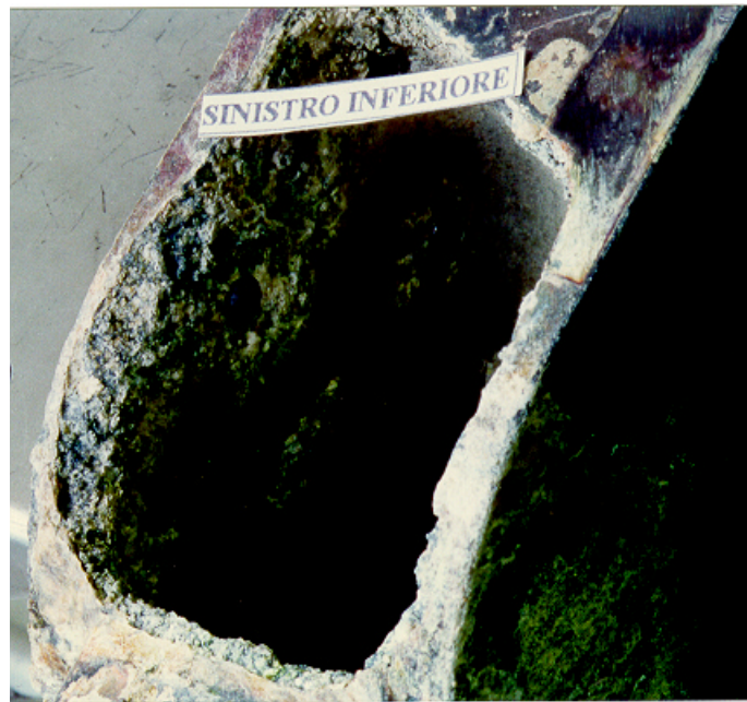
Fig. 9 – Galvanic Corrosion on a Mg Alloy Spacer, coupled with a steel beam in the MB-326 Central Section
