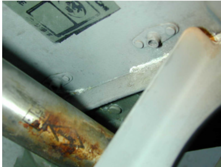
Fig. 11 – Galvanic Corrosion on the MB-339 Attach Fitting
