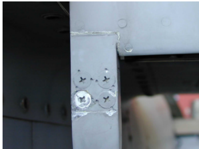
Fig. 10 – Galvanic Corrosion on the MB-339 between Mg Alloy Trim and Aluminum rivets
