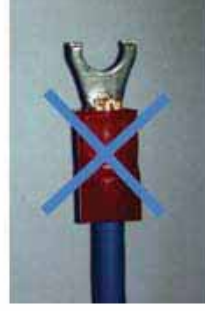
Terminal has been cut.
