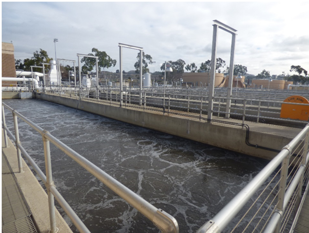
View of Aeration Tanks
