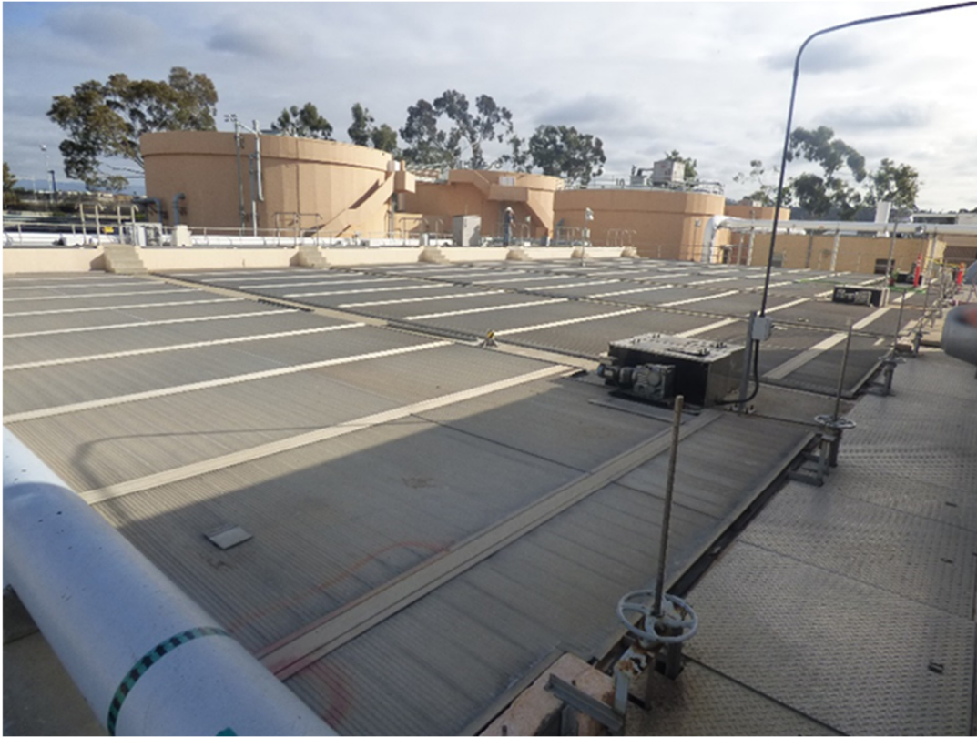
View of Primary Clarifiers (view to northeast with digesters in the background)
