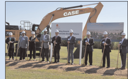
p54 First Solar Inc of Tempe, AZ, USA has broken ground its fifth fully vertically integrated factory in the USA, sited in Iberia Parish, Louisiana.
