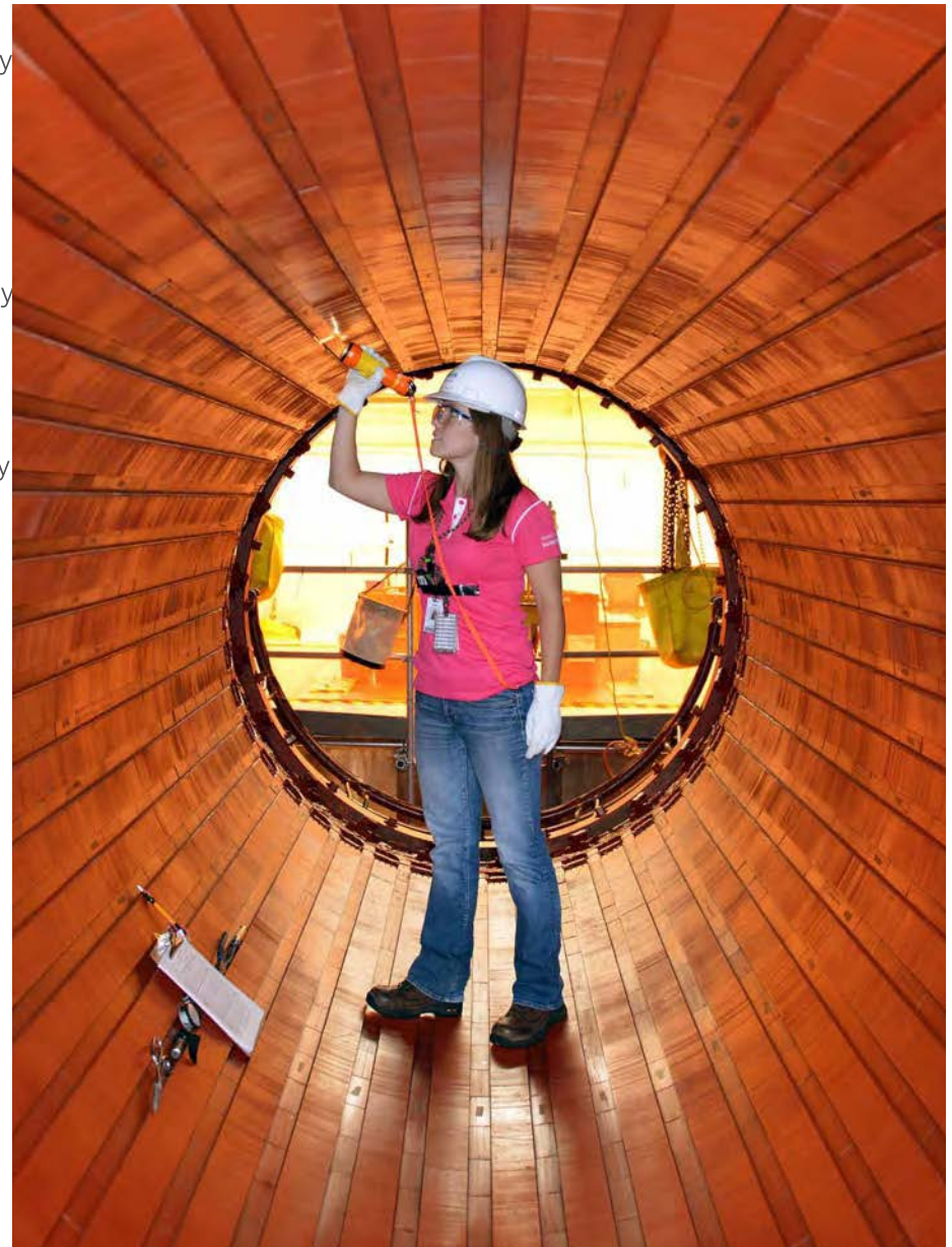
Inspecting power generation equipment at Byron Station.
