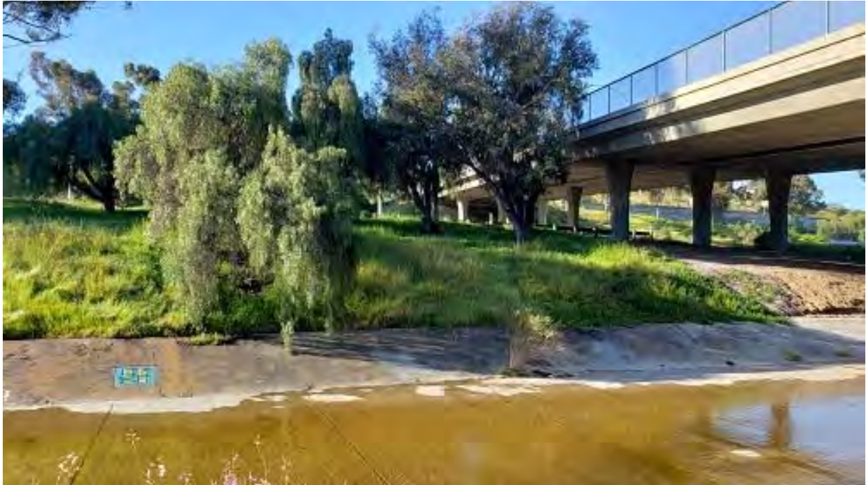
Photo 1. View of downstream-end of project near Home Ave. Concrete will remain for 200' upstream of Home Avenue Bridge. Eucalyptus woodland to south of Creek.
