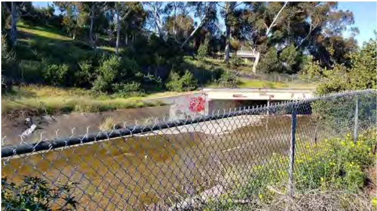
Photo 4. Old Federal Boulevard Bridge culvert will be removed, as well as the concrete in Chollas Creek.
