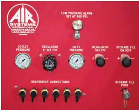
Custom cascade air control panels to manage entire fill system
