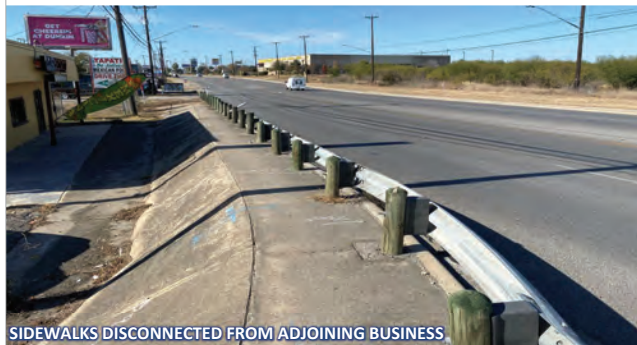
SIDEWALKS DISCONNECTED FROM ADJOINING BUSINESS
