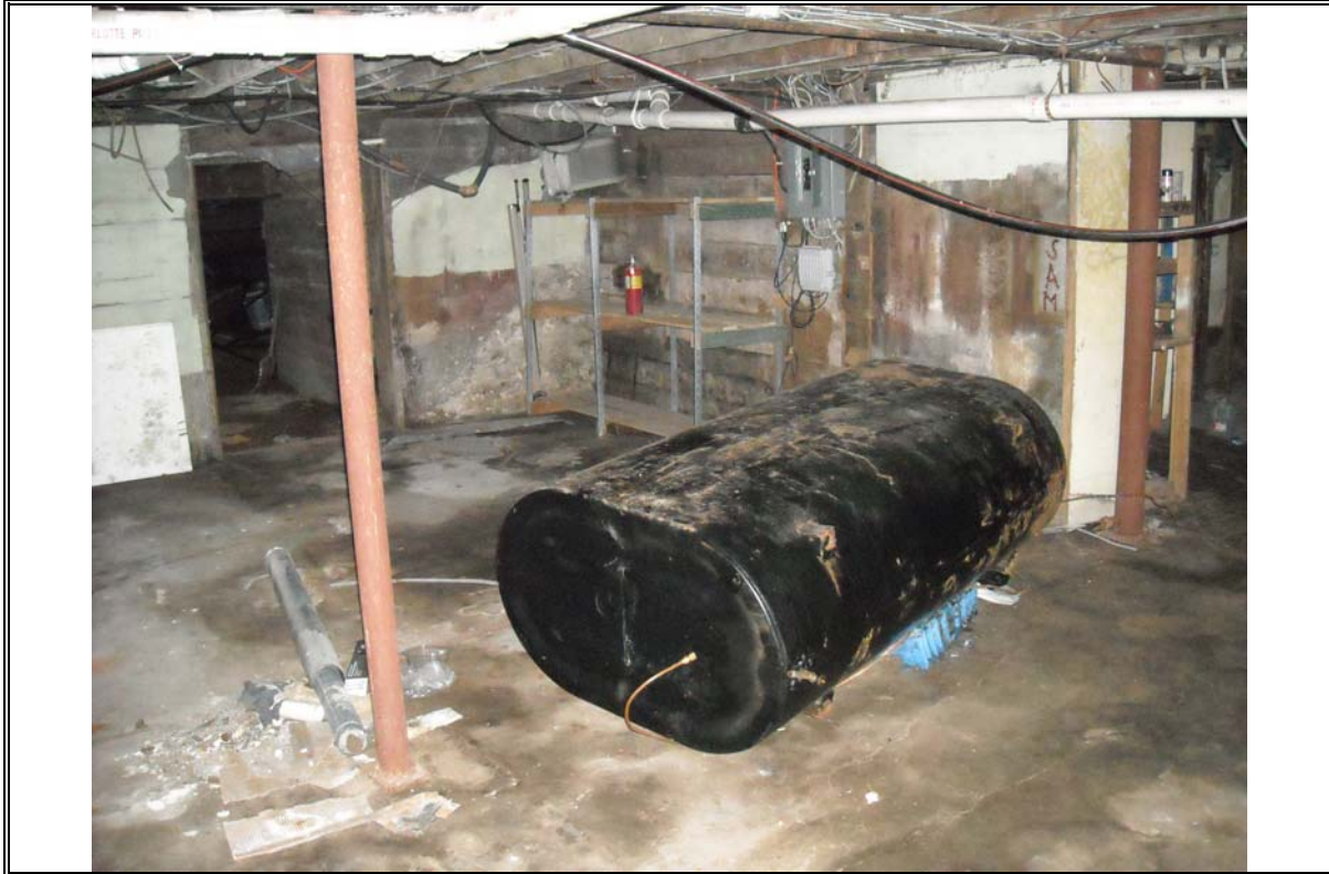
Photo 9: Abandoned heating oil tank observed in basement space at the north end of the Site building. No ground staining or odors were noted in the vicinity of the tank.
