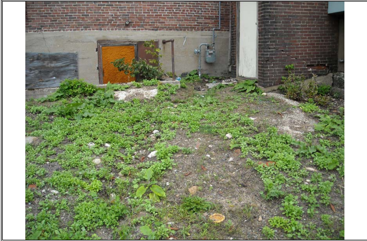
Photo 3: Gas line entering the back side of the Site building.
