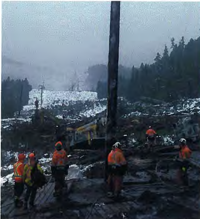
Our crews rebuild transmission pole structures that were damaged in a landslide.
