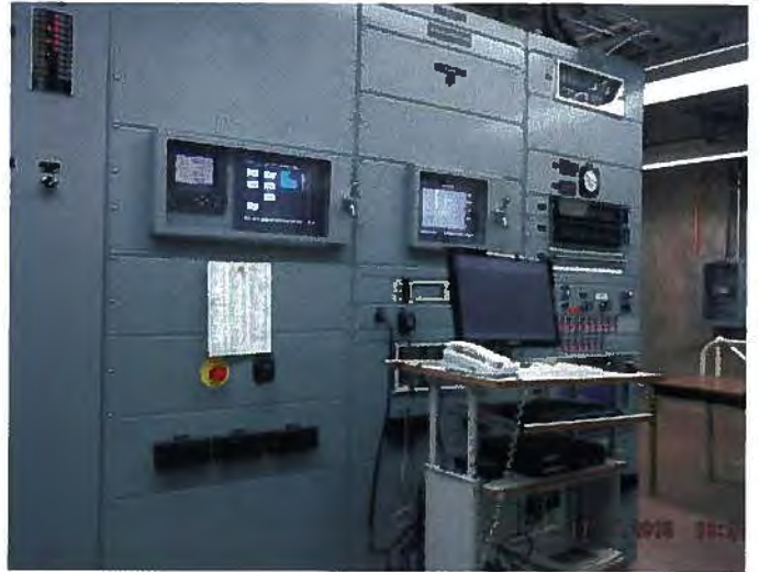
G5 unit control board – after.
