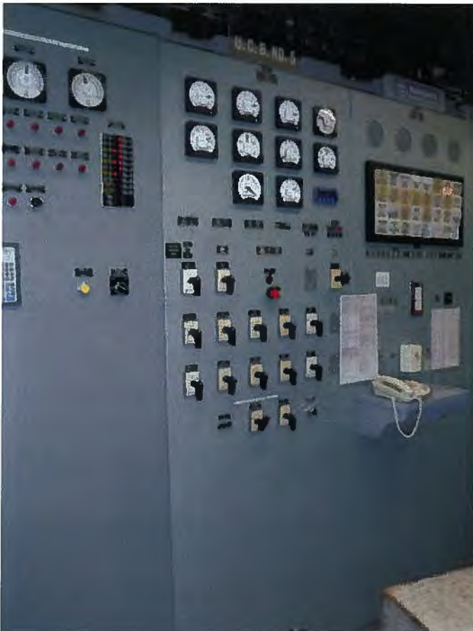
G5 unit control board – before.
