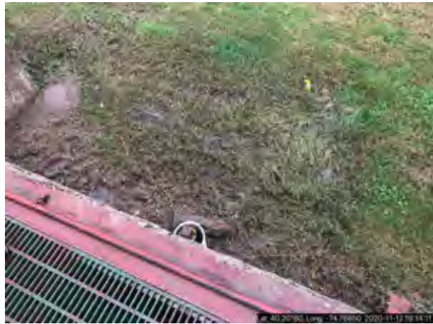
Photo #: Area of Sludge Overflow OM-11 4 O&M-0987403 A2 Description: Photo taken by BERNARD J KRASNISKY
