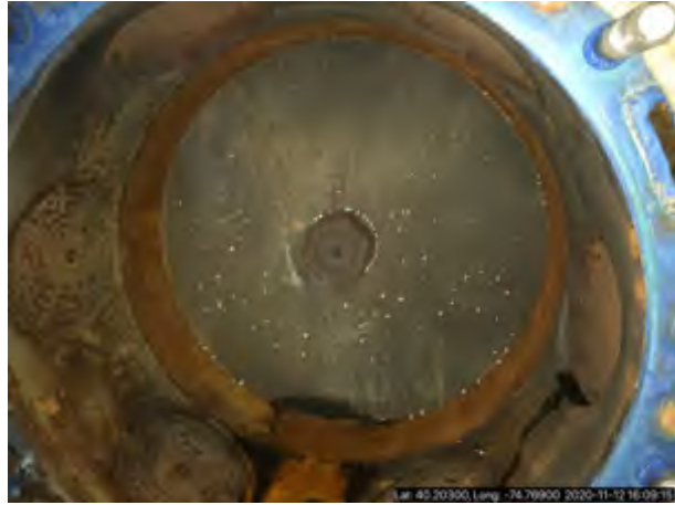
Photo #: Cracked North Unox Compressor OM-11 4 O&M-0987403 A2 Description: Photo taken by BERNARD J KRASNISKY
