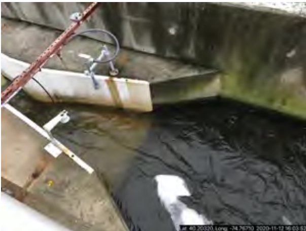
Photo #: Final Effluent TP-2 3 TP Treatment Plant-0987403 A2 Description: Photo taken by BERNARD J KRASNISKY
