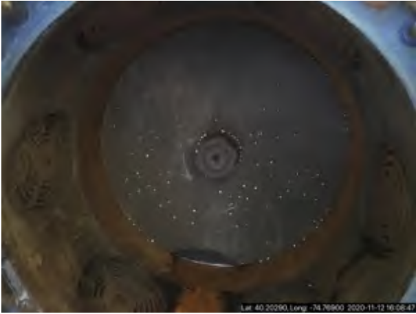
Photo #: Cracked Compressor OM-11 4 O&M-0987403 A2 Description: Photo taken by BERNARD J KRASNISKY
