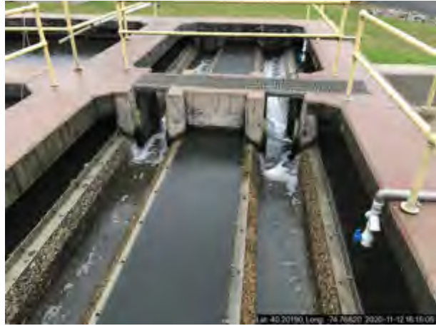
Photo #: South Plant Secon Secondary Weirs OM-11 4 O&M-0987403 A2 Description: Photo taken by BERNARD J KRASNISKY
