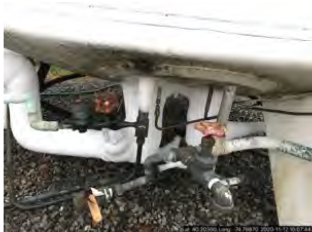
Photo #: Repaired O2 tank line OM-11 4 O&M-0987403 A2 Description: Photo taken by BERNARD J KRASNISKY
