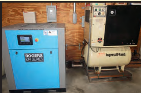
15 HP INGERSOLL RAND AND 20 HP ROGERS ROTARY SCREW AIR COMPRESSORS
