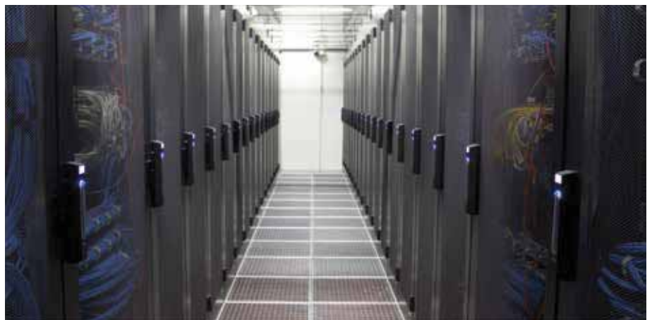
@lock solution with MLR handles in a co-location datacenter
