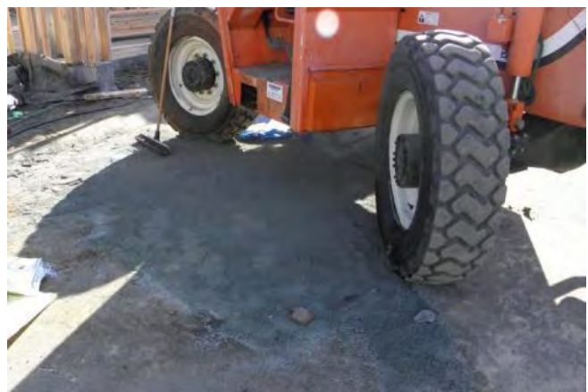
Figure 18: Hydraulic hose leak and absorbent deployment
