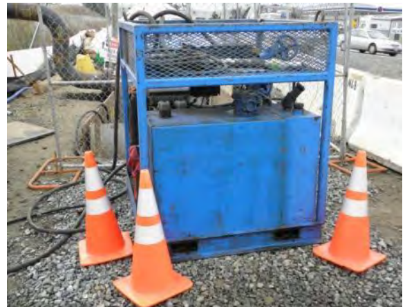
Figure 20: Hydraulic tank leaking onto ground
