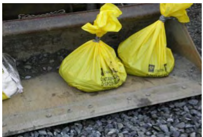
Figure 16: Contaminated soil properly prepared for disposal
