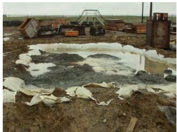
Figure 10: Poorly located, installed, and maintained
