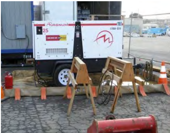
Figure 19: Generator on secondary containment
