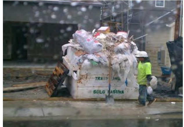
Figure 14: Overused and improperly covered during rain
