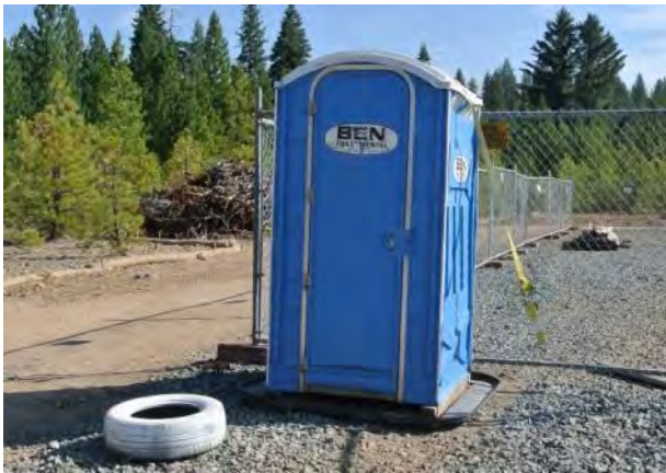
Figure 11: Properly placed on tray and tied down
