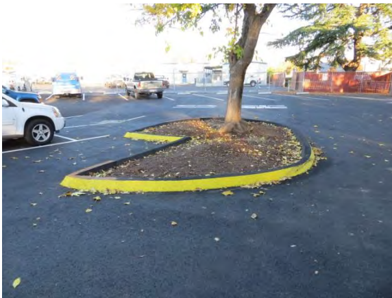
Planter area in need of soil stabilization
