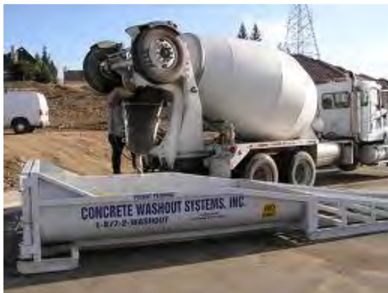
Concrete washout system
