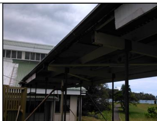
Figure 21.2 Walkway not repaired
