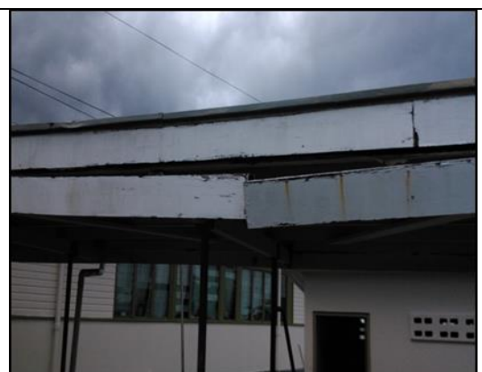
Figure 21.3 Repair on roof not done
