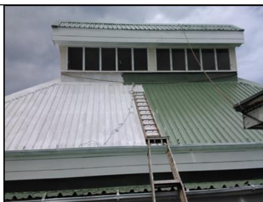
Figure 21.4 Roof of the Library not repaired
