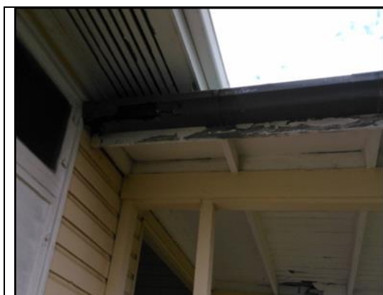
Figure 21.1 Gutters and Ceiling not Repaired
