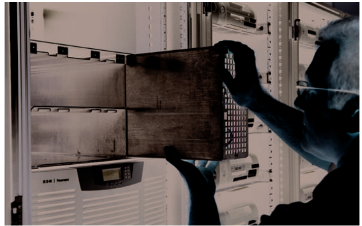
IT staff can easily install electronics modules.
