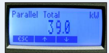
Display full system output from any UPS
