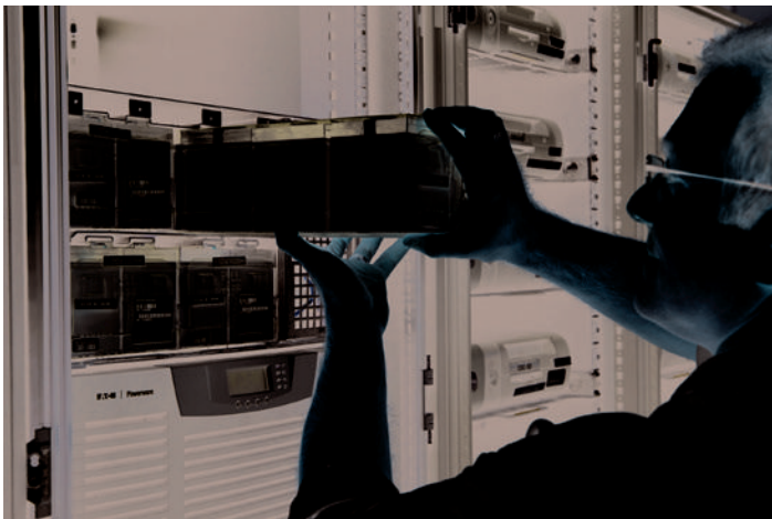
IT staff can easily replace battery modules.
