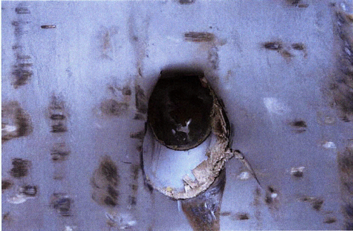
Figure 3.5-23 – LP1 Puncture Bar Damage after Removal of Bar
