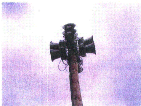
Figure 4 ATI omni-directional siren system mounted at the GTRI outdoor test facility.
