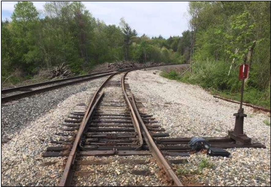
6c. Double Switch Point Derail
