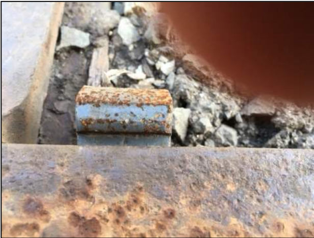
Tie Plate with Anchors Overdriven
