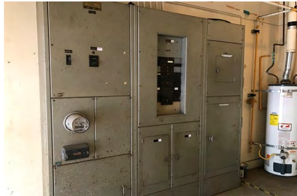
#34 SWITCHBOARD, 800 AMP, REPLACE
