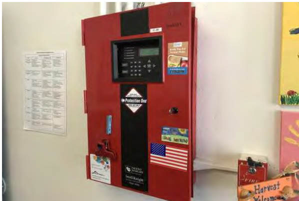
#35 FIRE ALARM CONTROL PANEL
