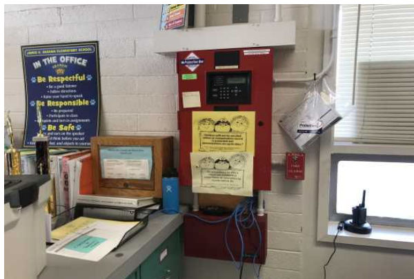
#47 FIRE ALARM CONTROL PANEL
