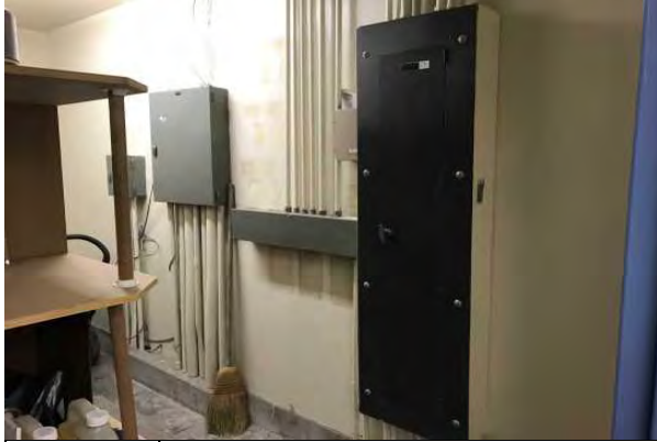
#55 ELECTRICAL DISTRIBUTION SYSTEM
