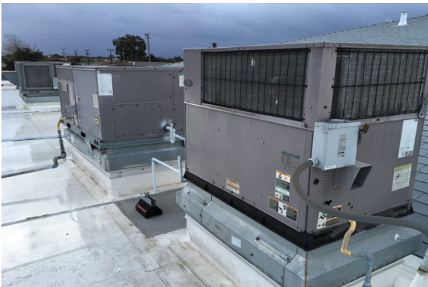
#17 HVAC ROOF MOUNTED UNIT 4
