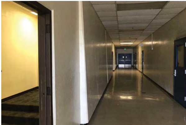
#47 BATTERED CAST CONCRETE WALLS, BUILDING 300
