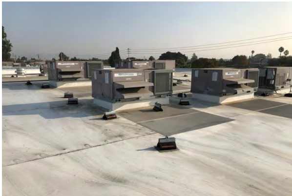
#33 CLASSROOM BUILDING HVAC
