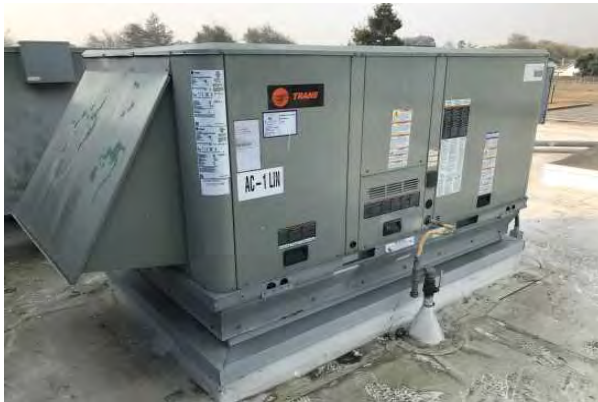
#45 HEAT PUMP, PACKAGED (RTU)
