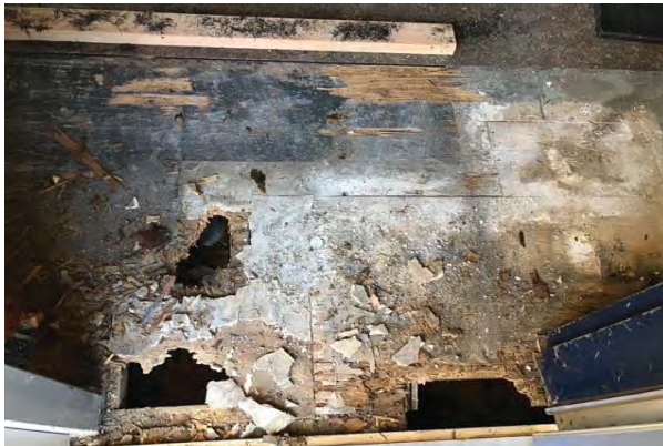
#29 ROTTING SUBFLOOR, WEIGHTLIFTING BUILDING
