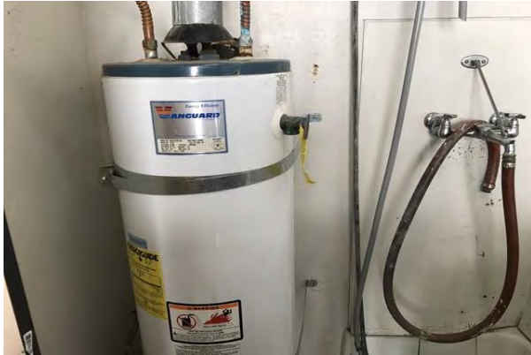
#37 WATER HEATER, GAS
