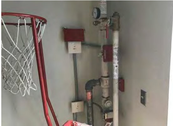
#43 SPRINKLER SYSTEM - STAGE
