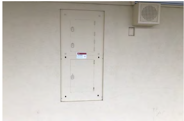
#30 OLD DISTRIBUTION PANEL
