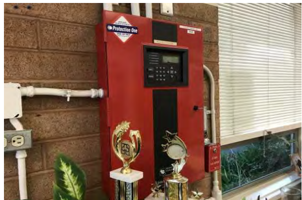
#42 FIRE ALARM CONTROL PANEL
