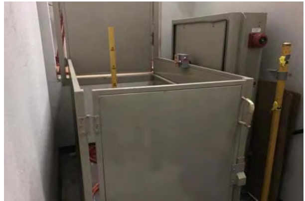
#34 BUILDING 6 - WHEELCHAIR LIFT
