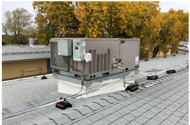
#18 PACKAGED UNIT (RTU), UNIT 3
