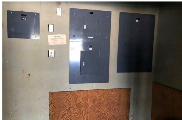
#46 CLASSROOM ELECTRICAL DISTRIBUTION
