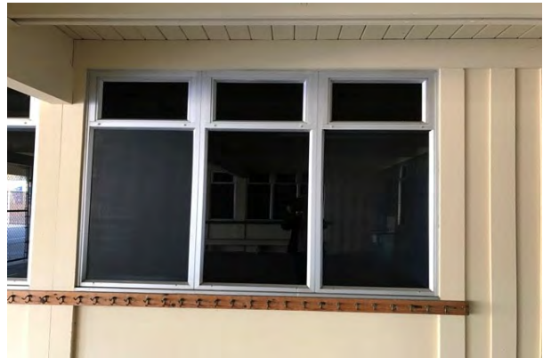
#28 TYPICAL ALUMINUM WINDOWS
