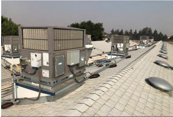
#31 HVAC AT BUILDINGS 1, 2 AND 3
