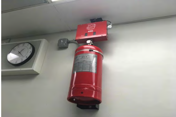
#55 FIRE SUPPRESSION SYSTEM, KITCHEN (CO2)
