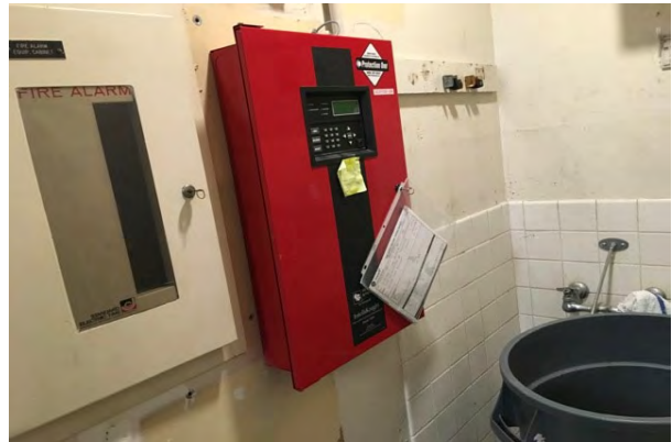
#34 FIRE ALARM PANEL WHITEFORD BUILDING
