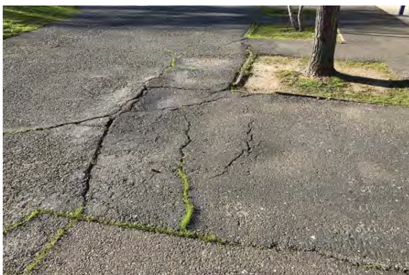
#23 UNEVEN WALKING SURFACE
