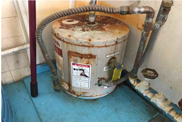
#37 DAMAGED CLASSROOM WATER HEATER
