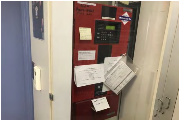
#39 FIRE ALARM CONTROL PANEL
