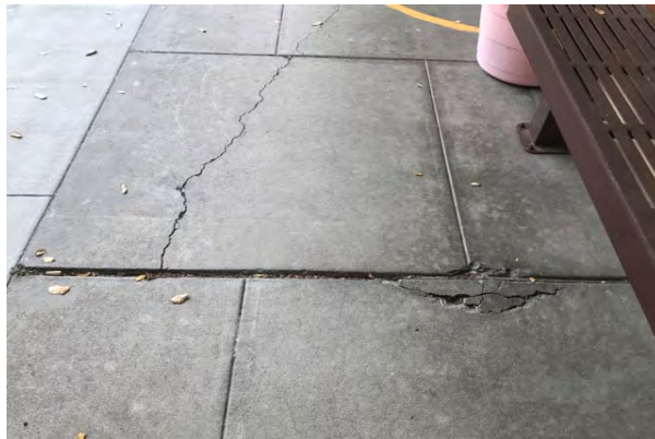
#17 CRACKING AND UPLIFT SEEN AT MUCH OF THE FLATWORK
