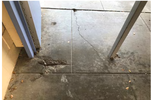
#16 CRACKING AND UPLIFT SEEN AT MUCH OF THE FLATWORK
