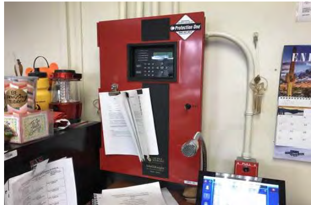
#52 FIRE ALARM CONTROL PANEL
