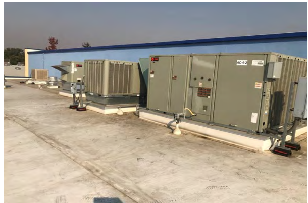
#30 HVAC AT THE MULTIPURPOSE BUILDING
