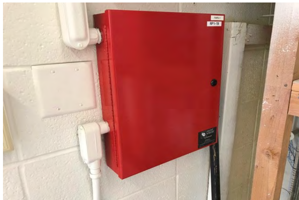
#45 FIRE ALARM CONTROL PANEL
