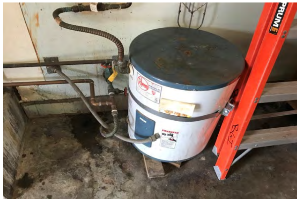
#39 WATER HEATER, ELECTRIC
