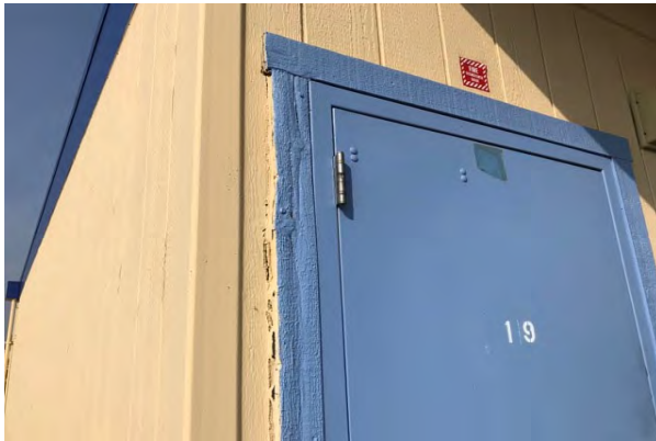
#27 ROTTING TRIM AND CAULKING CRACKS AT PORTABLE BUILDING DOOR
