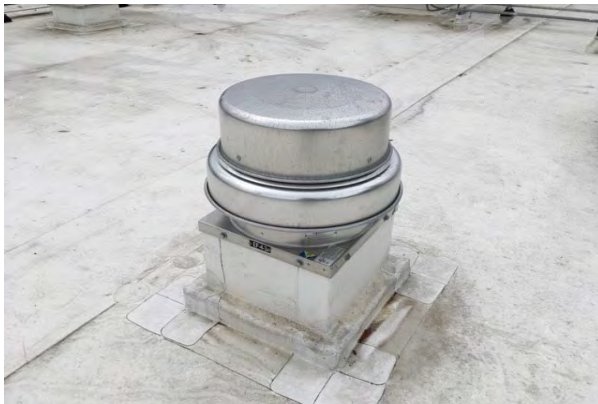
#11 ROOF MOUNTED EXHAUST FAN
