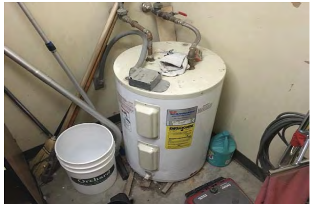
#52 ELECTRIC WATER HEATER
