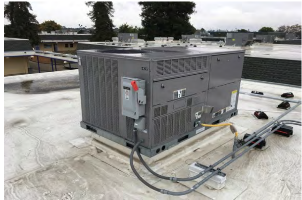
#10 PACKAGED UNIT (RTU)
