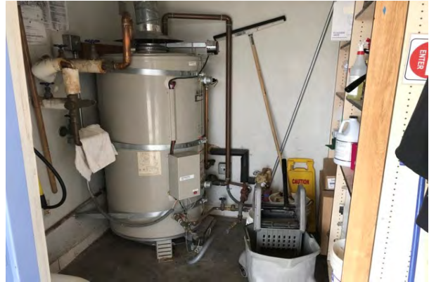
#38 MULTI PURPOSE ROOM WATER HEATER
