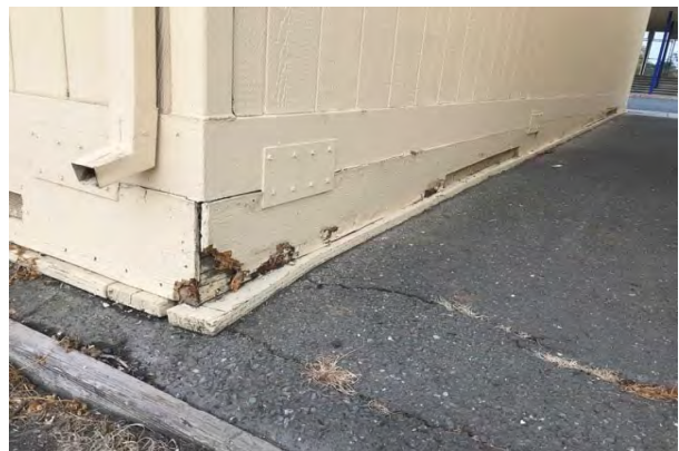
#24 EXTERIOR WALL DETERIORATION AT PORTABLES
