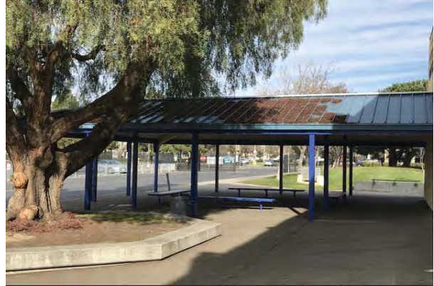
#20 TREE TRIMMING NEEDED
