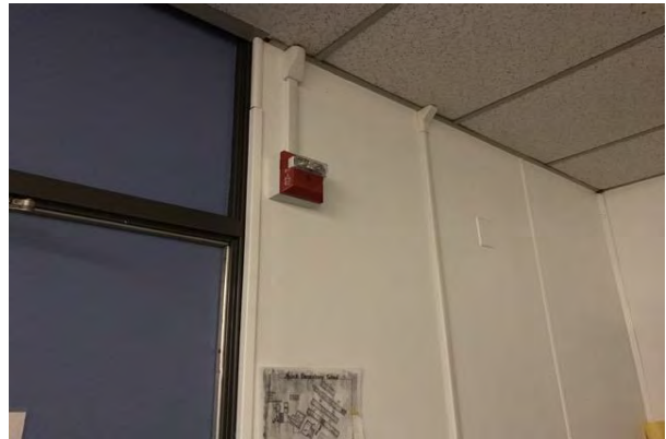
#40 FIRE ALARM SYSTEM
