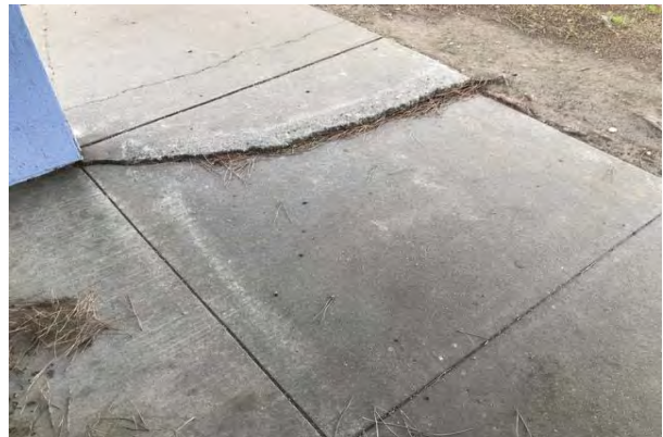
#22 UNEVEN WALKING SURFACE
