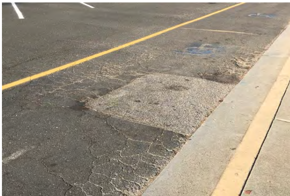
#9 PARKING LOT DAMAGE
