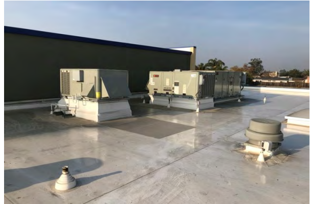
#32 MULTI PURPOSE BUILDING HVAC
