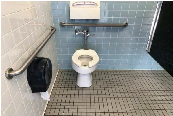
#41 TOILET, TANKLESS (WATER CLOSET)
