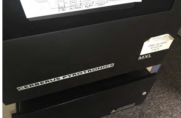
#56 FIRE ALARM SYSTEM
