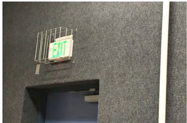
#46 EXIT LIGHTING FIXTURE
