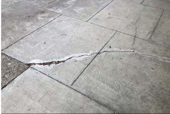
#13 CONCRETE WALKWAY, TRIP HAZARD
