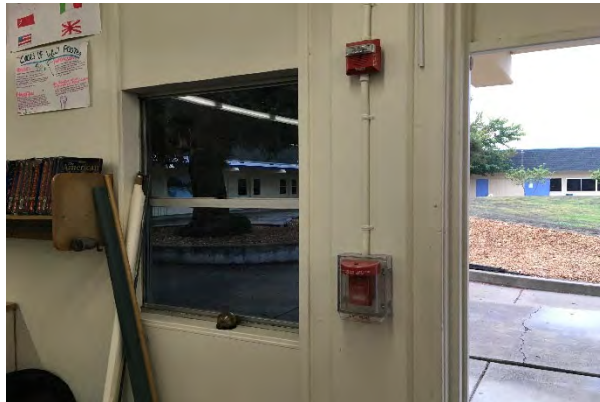
#33 FIRE ALARM SYSTEM
