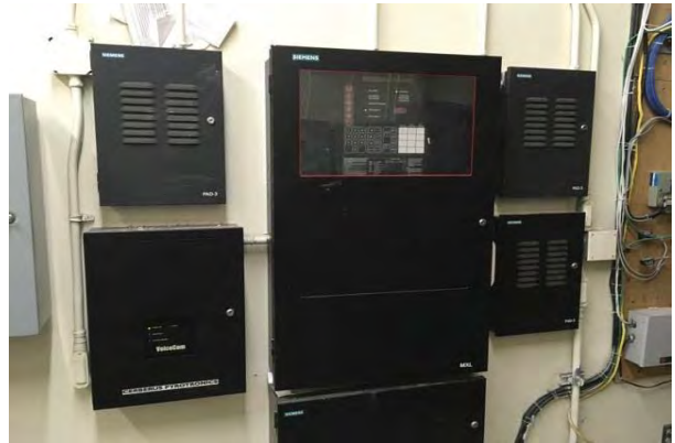
#60 FIRE ALARM CONTROL PANEL
