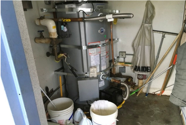
#31 HOT WATER HEATER
