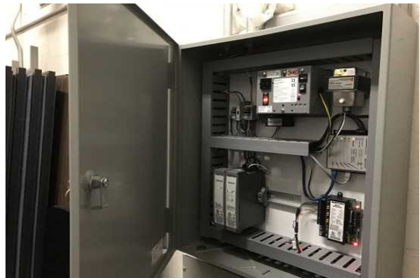
#46 BUILDING AUTOMATION SYSTEM (BAS)
