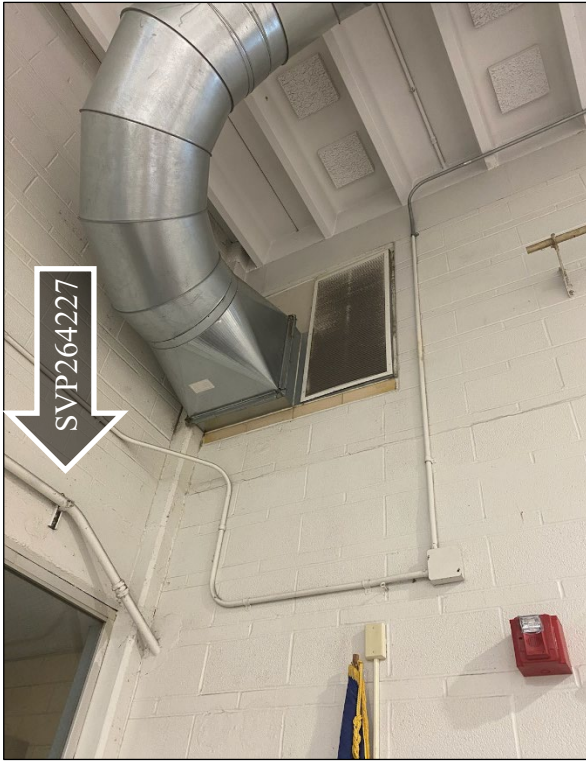
Image 3. STSU3-UB6 (dust on top of conduit piping)
