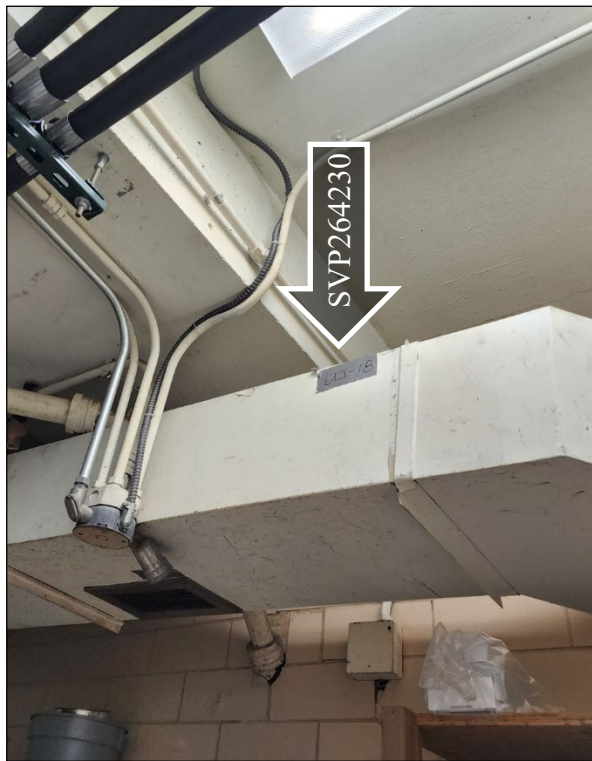
Image 6. STSU3-UB18 (dust on top of ducting)
