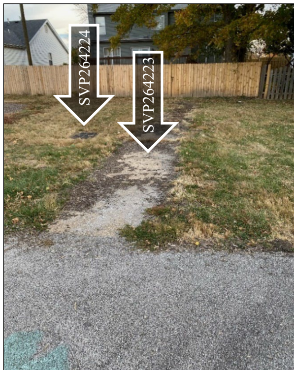
Image 10. Pavement Sediment Near Basketball Courts
